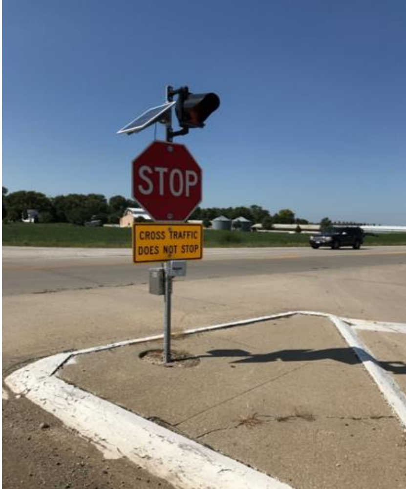
Figure 3-10: Flashing beacon installed at one of the treatment sites
