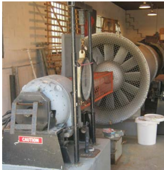
Figure 6.2. Main fan infrastructure at Experimental Mine
