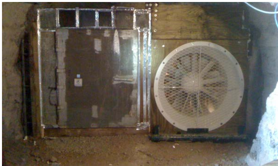
Figure 7.18. East booster fan installed in bulkhead
