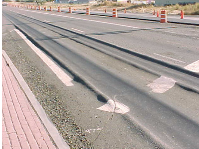
Figure 2.19 - Permanent deformation (rutting)
