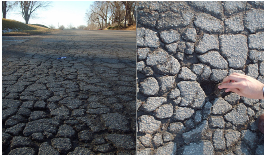
Figure 2.17 - Fatigue damaged pavement in Lincoln, NE
