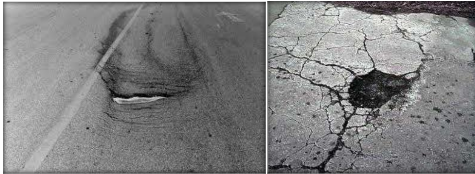
Figure 1: Potholes formed due to excessive fatigue cracking and permanent deformation.
