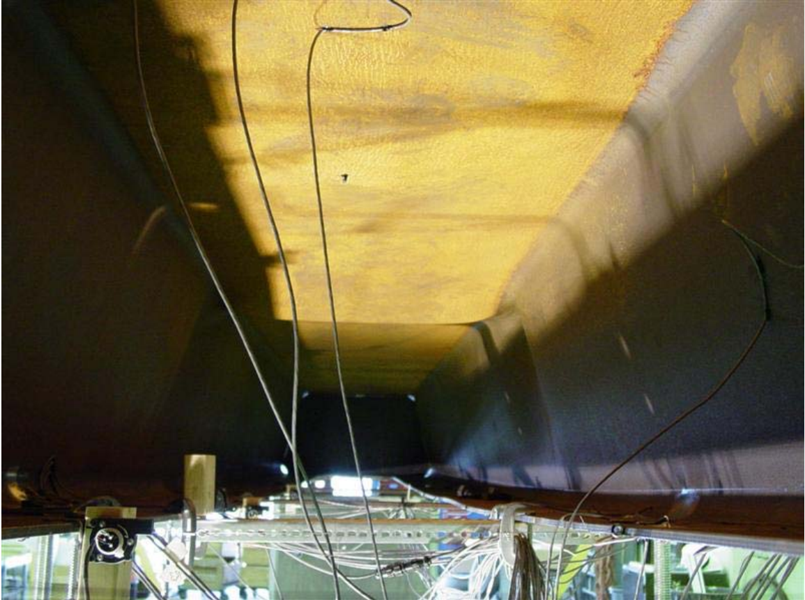
Figure 3-10 Inside of folded plate girder after failure
