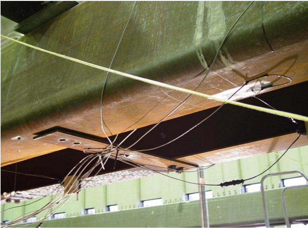
Figure 2-13 Disconnected tie plate at section H
