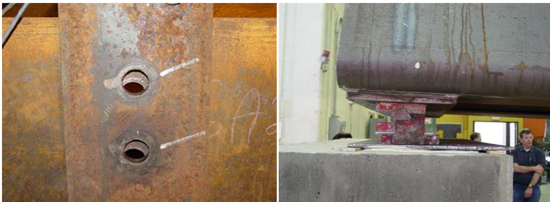
Figure 3-17 (left) Flange and tie plate bolt hole alignment after loading, (right) girder movement at support.
