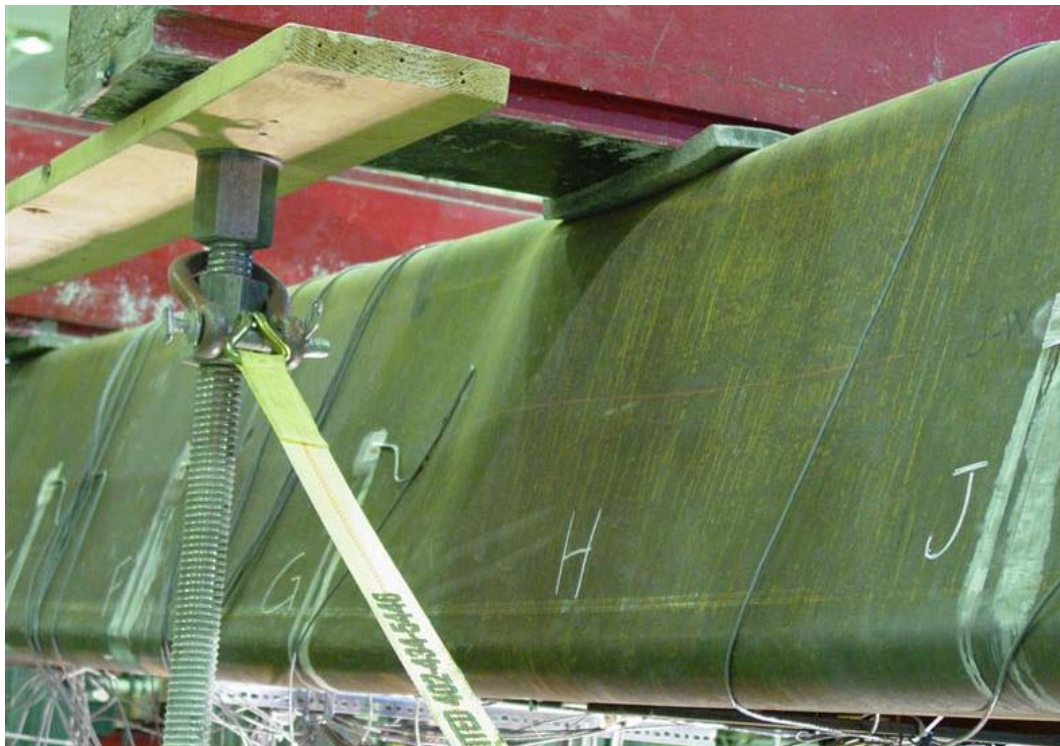
Figure 3-9 Web deformation from loading.
