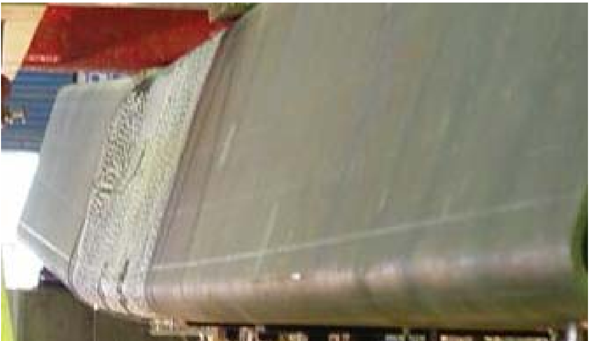
Figure 3-12 North side of girder facing east showing girder deflection and web buckling
