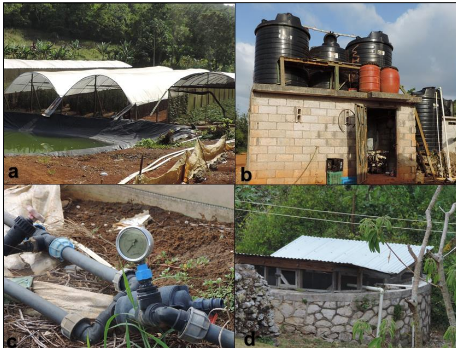
Figure 4.5 Water management options: a. Water harvesting pond; b. Black tank; c. Greenhouse drip system connected to with a metered connection to government irrigation line; d. Concrete tank
