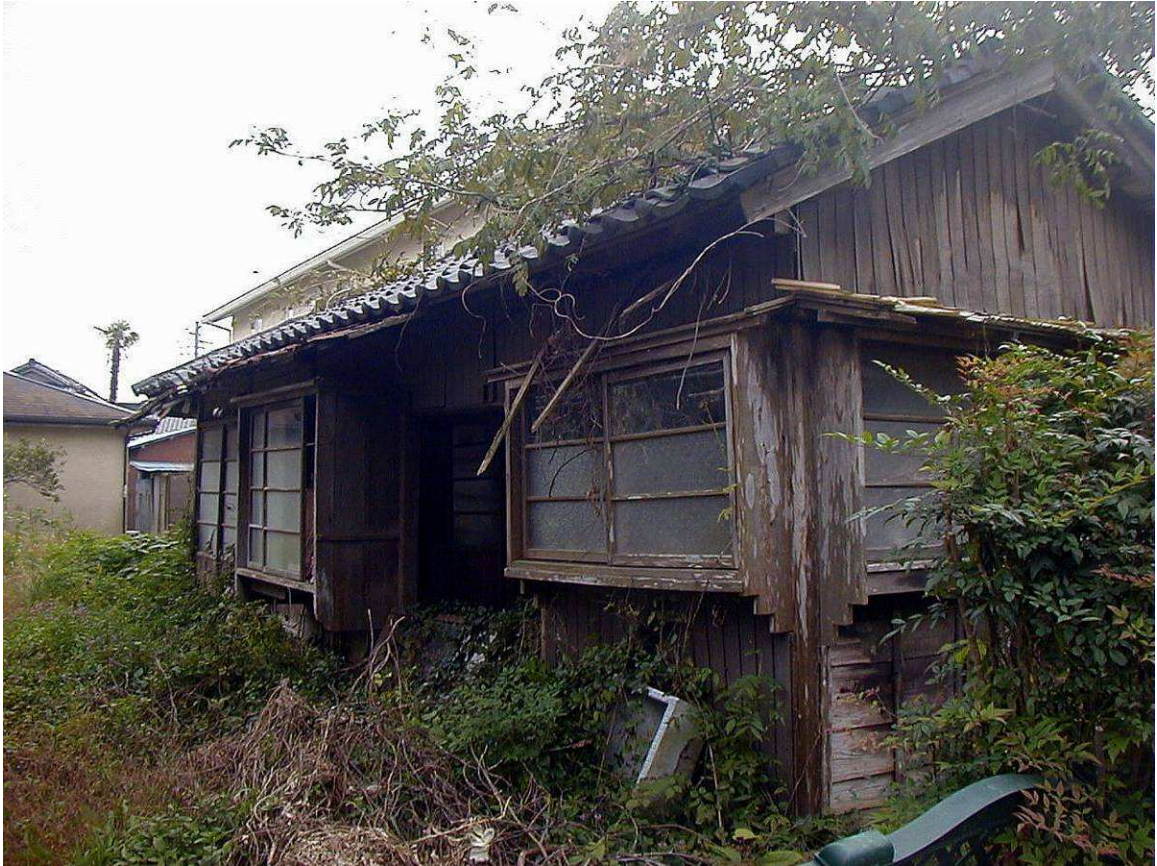
Fig.2.1:Redundancy and processes of physical decay. In the humid Kanto climate unmaintained and vacant wooden structures deteriorate within three to five years. Naruto-machi, Sanmu-shi .
