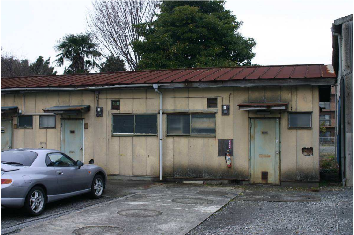
Fig. 7.12. One form of 'nagaya' tenement dwelling used for 'issued accommodation' by a joinery firm in Murata in the 1960's, now storage. It is very difficult to piece together any overview of this kind of dwelling at the period because it was almost all demolished by 1990.
