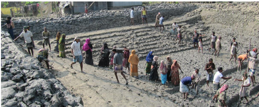
Figure 3.2: A Water Tank Digging Work under a ‘Cash for Work’ Project, where Men and Women are Working Together (Source: Author, 10/11/2009).
