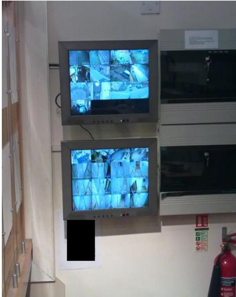
Figure 10 CCTV system at BP
