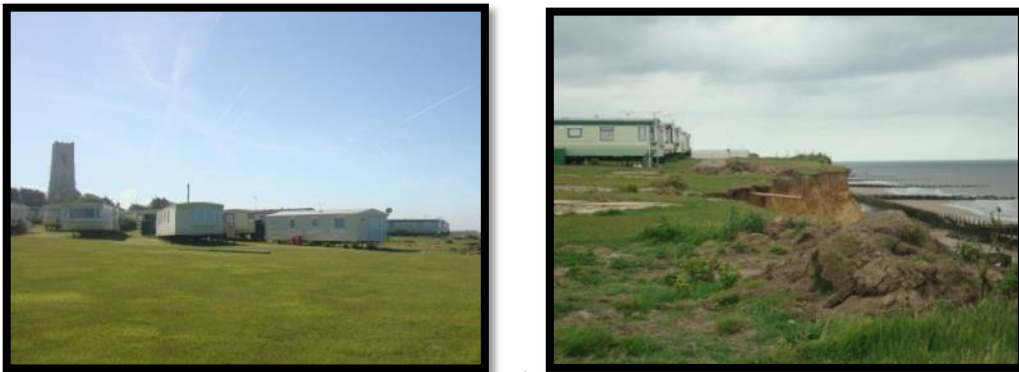
a) b) Figure 85: Photos of 'Bottom Field' Happisburgh - a) Photo showing the proximity of Happisburgh church to the erosion, b) Evidence of the retreat of the caravan park
