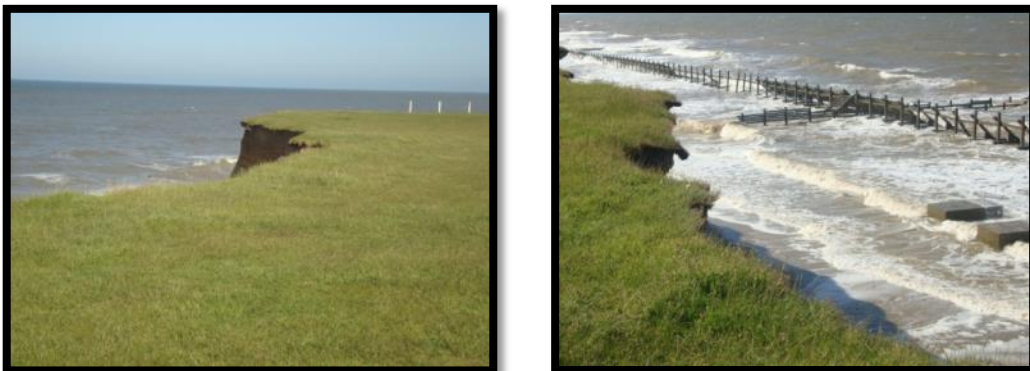
a) b) Figure 86: Bottom field photos: a) Location of the former stairs to the beach, b) Overhanging grass at the cliff edge and the concrete blocks where the stairs to the beach were under two years previously.
