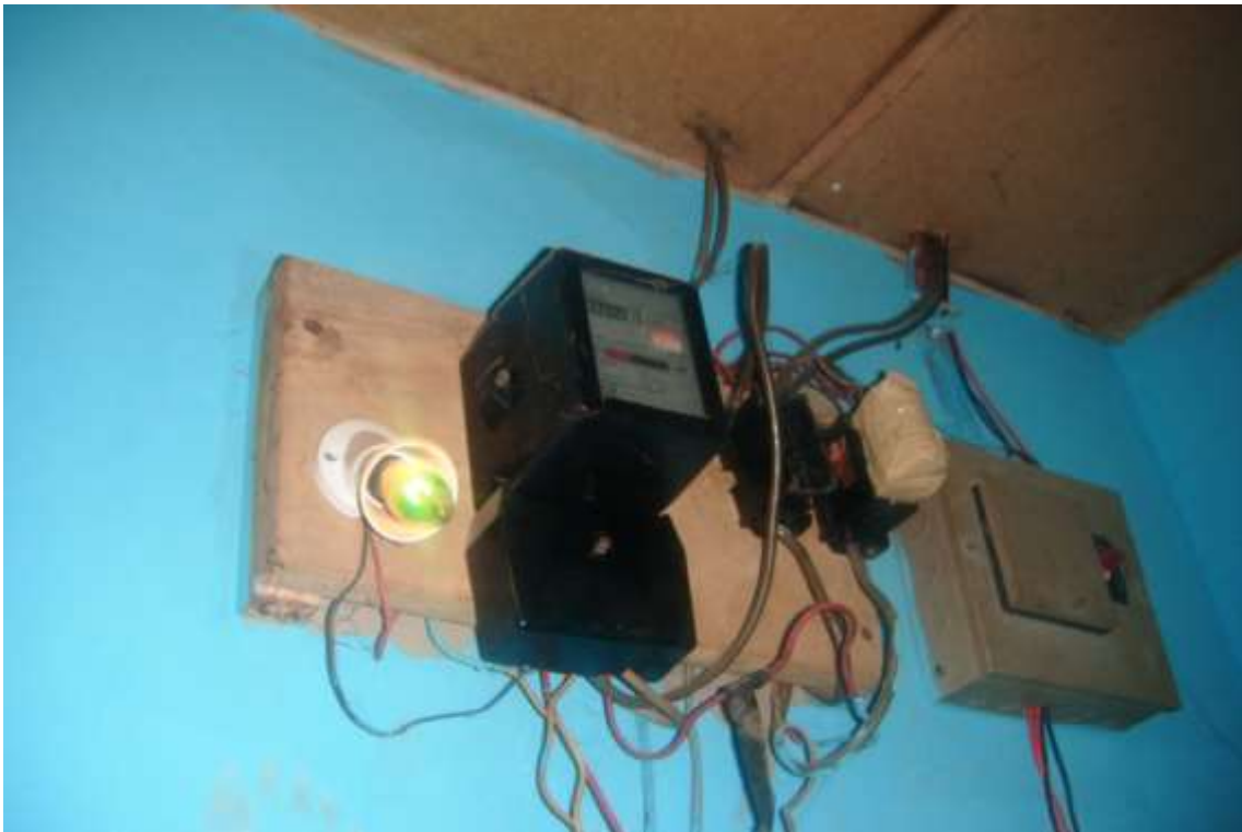
Plate 3.8: A typical credit/electromechanical meter connection Source: Fieldwork (2012) - Permission granted by household for photograph to be taken
