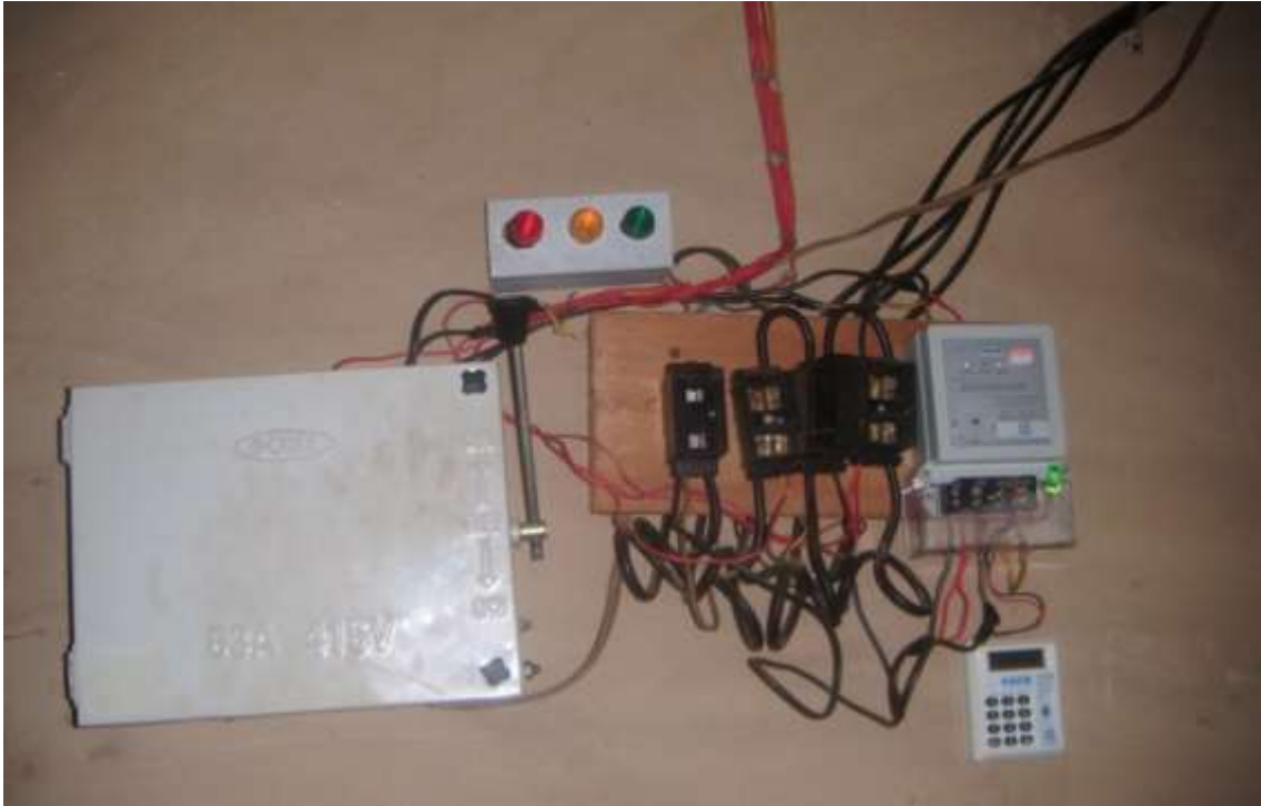
Plate 3.7: A typical single-phase prepayment meter connection Source: Fieldwork (2012) - Permission granted by household for photograph to be taken
