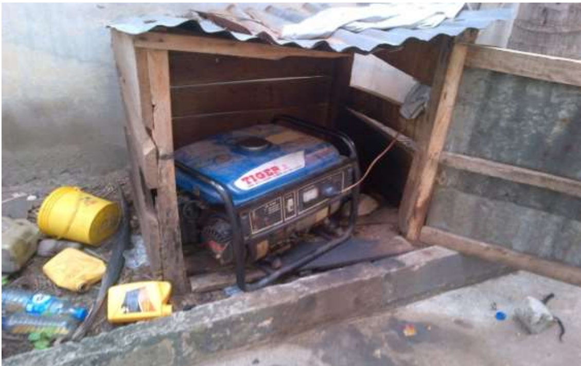
Plate 5.2: A typical 2.5KVA type of generator (TG950) Source: Fieldwork (2012)
