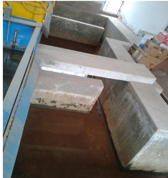
Figure 3.8. Photo of Volumetric tank
