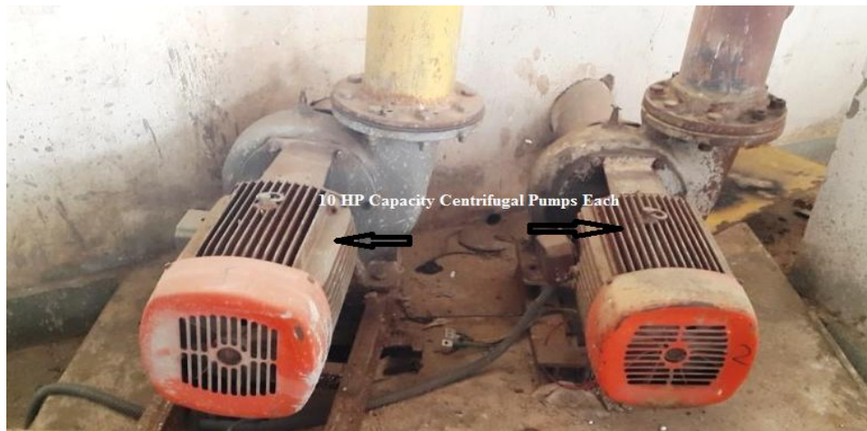
Figure 3.2: Photo of Centrifugal Pumps (10HP capacity each)
