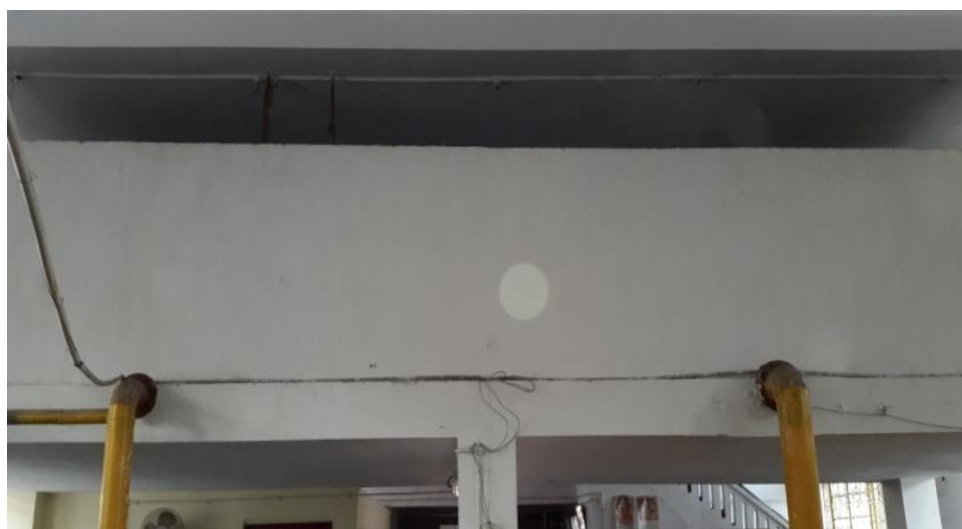
Figure 3.3: Photo of Overhead Tank
