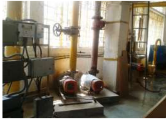
Fig 3.4 Two parallel pumps
