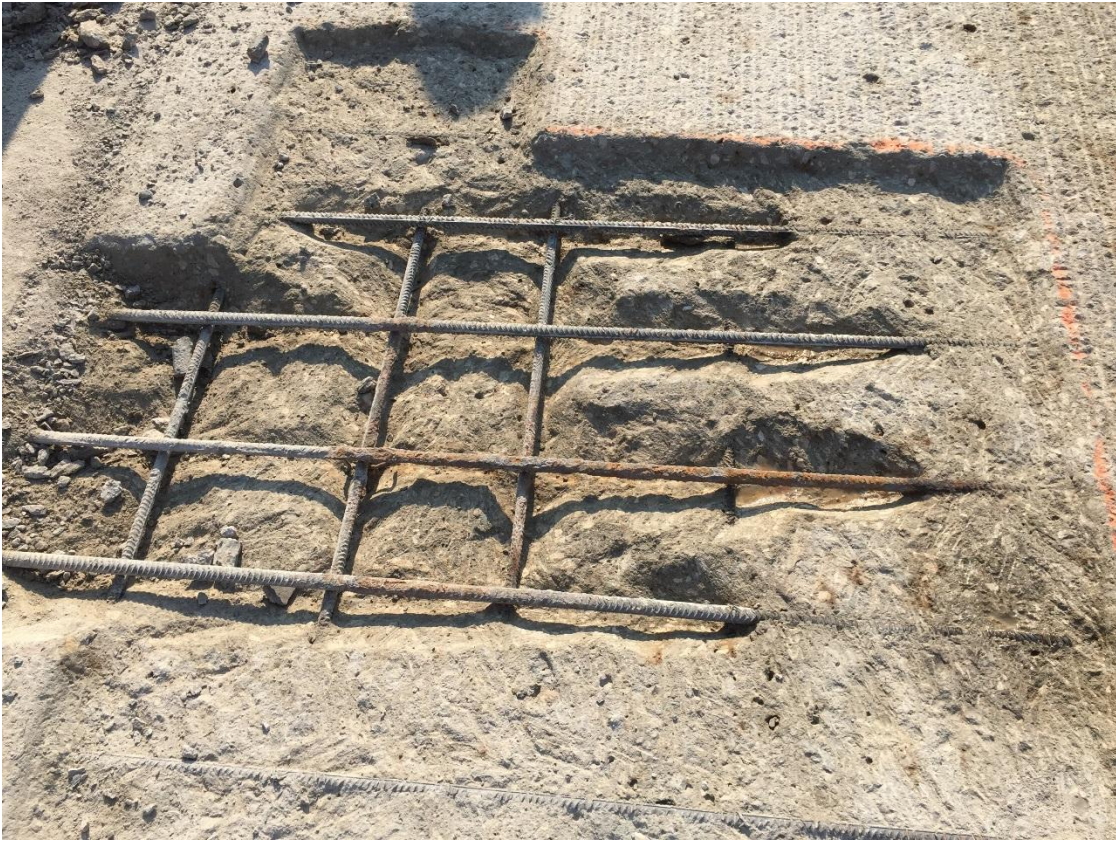
Figure 44. Deteriorated area of the deck after removal of the substrate concrete
