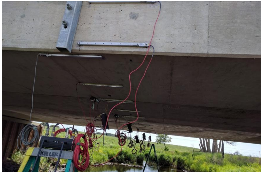
Figure 28. Instrumentation mounted on the bridge
