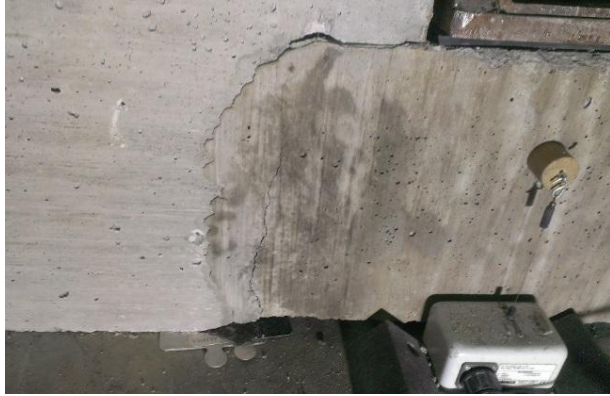
a) Propagation of crack
