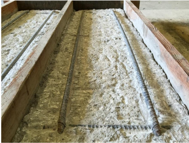
Figure 96. Negative bending flexural test specimen after concrete removal to required depth (Case 3)
