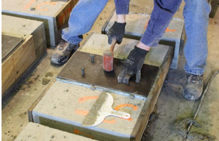
Figure 53. Tapping the steel plate to embed the shear studs on a pull-off test specimen
