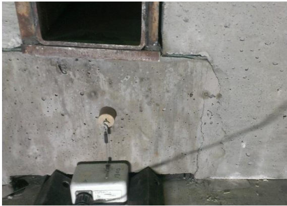
a) Propagation of crack
