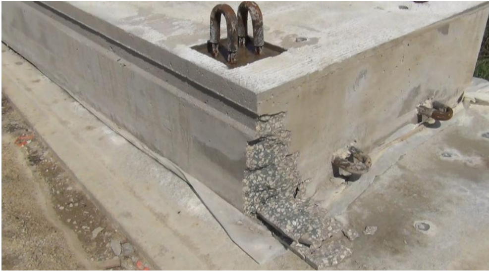
Figure 14. Concrete spalling on non-pulling side of the beam
