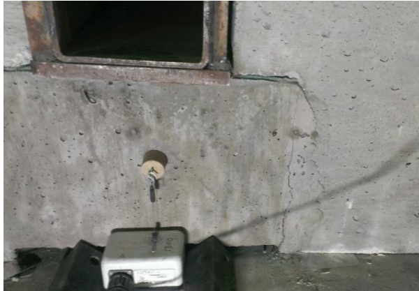
a) Propagation of crack
