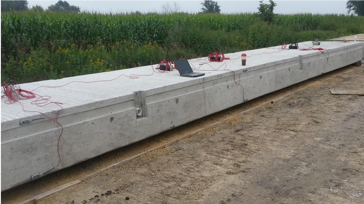
Figure 16. Installed strain gage and data collection system for lift/move
