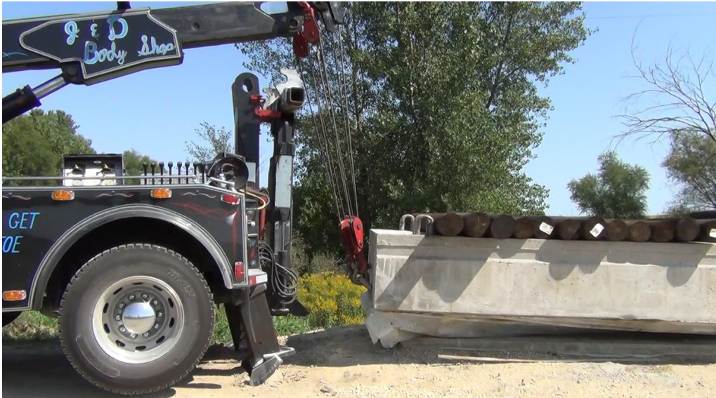
a) Beam lifted by tow truck
