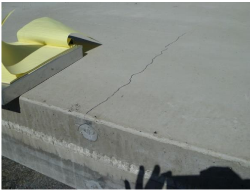
Figure 2.7 Top layer of longitudinal prestressing strand splitting failure
