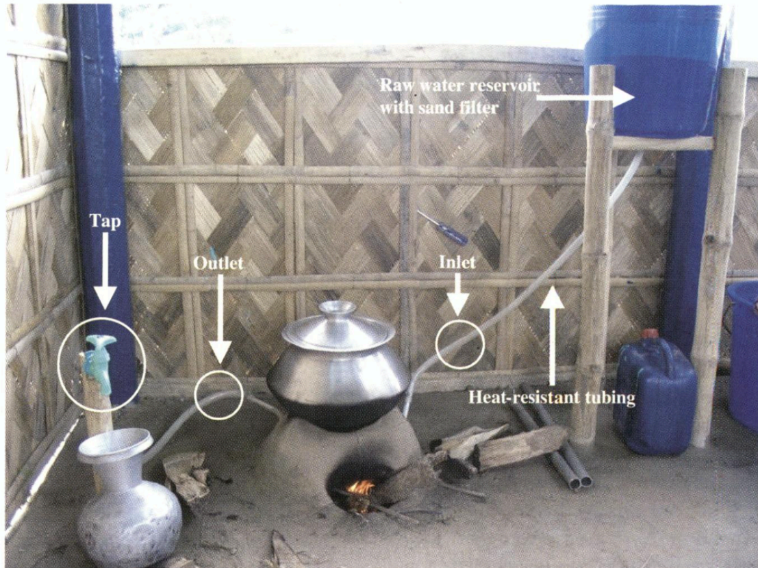
Figure 8: Overview of the entire chulli system (reprinted with permission of JSTOR) (Islam et. al., 2006)
