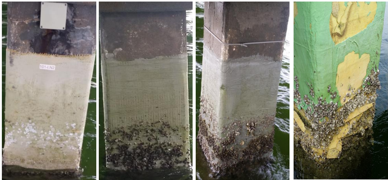
Figure 10.4 Photos of FRP repairs in piles. (left to right) 101 B, 101C, 103C and 104B
