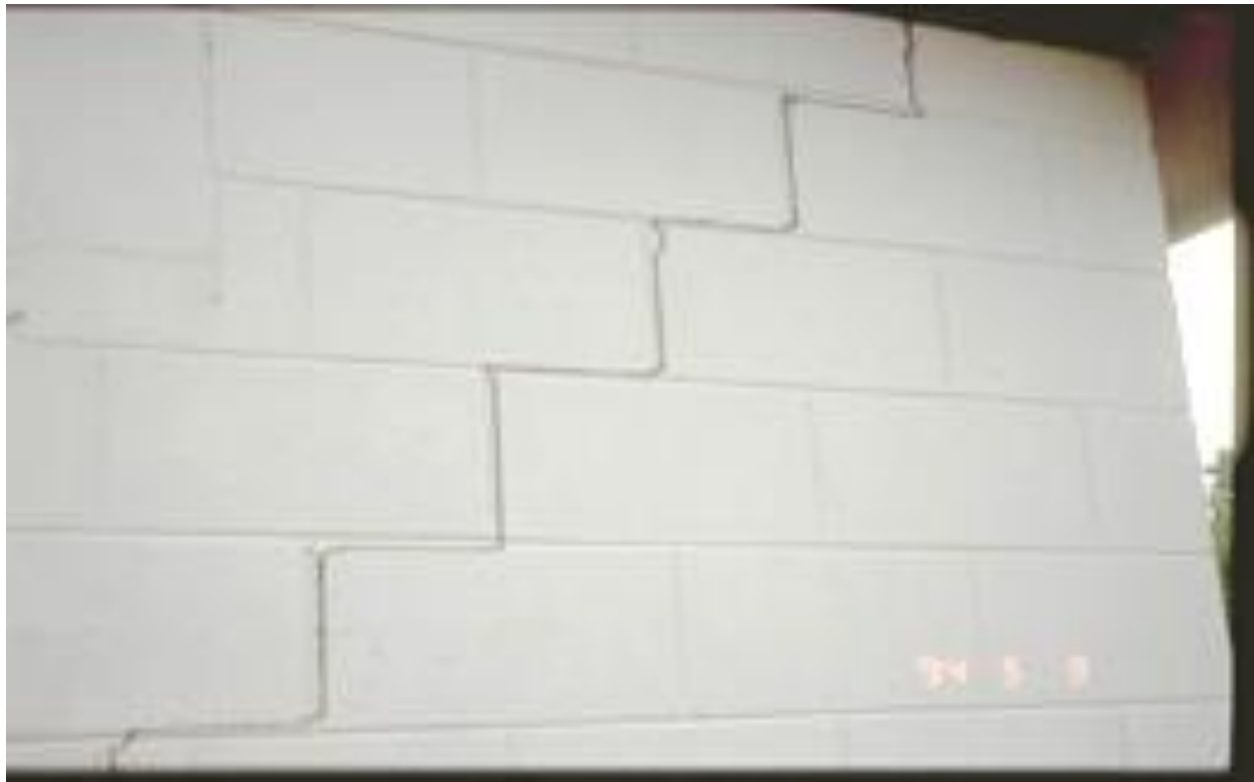
Figure 9.1 Characteristic stair-step cracking in CMU wall.
