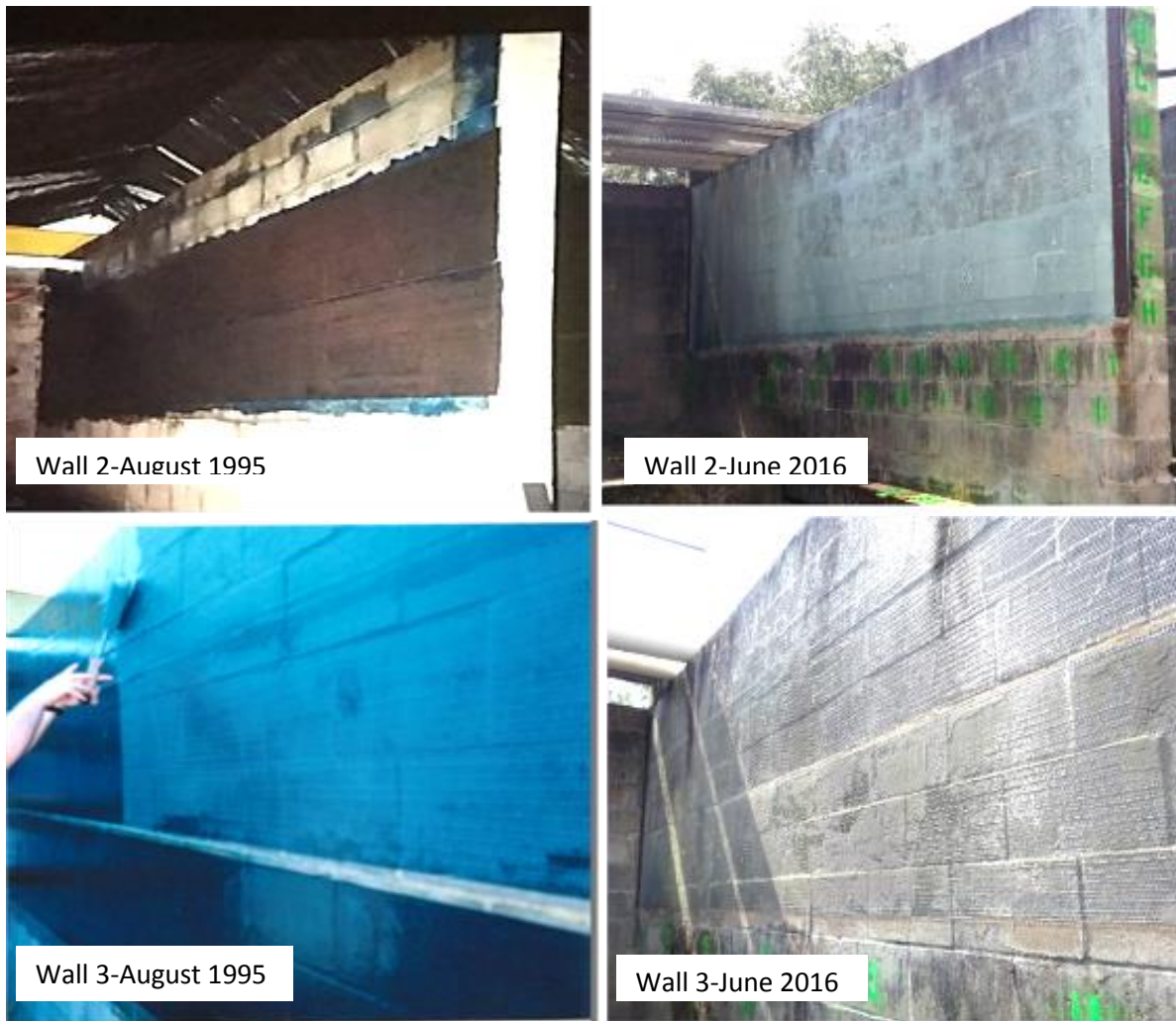
Figure 9.7 Comparison of images for wall 2 and wall 3. At installation and after exposure
