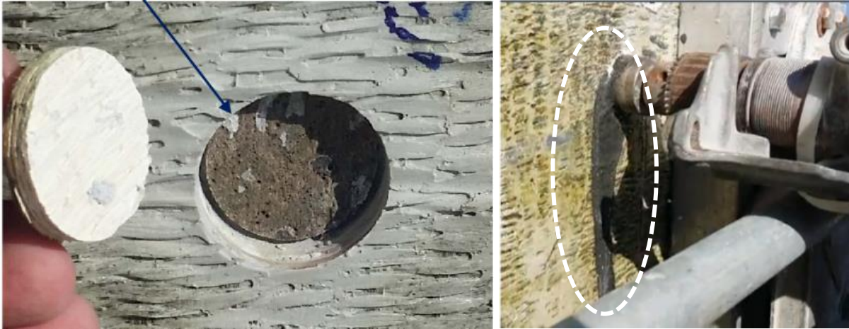
(a) Moisture in bond plane and between FRP layers
