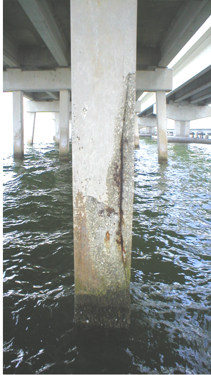
Figure 1.3 Corroding steel in one bent pile in east bound Gandy Bridge (built circa 1970).
