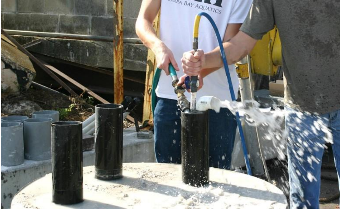
Figure 4.10. Airlift vacuum used to clean up fragments from inside the installed casings.
