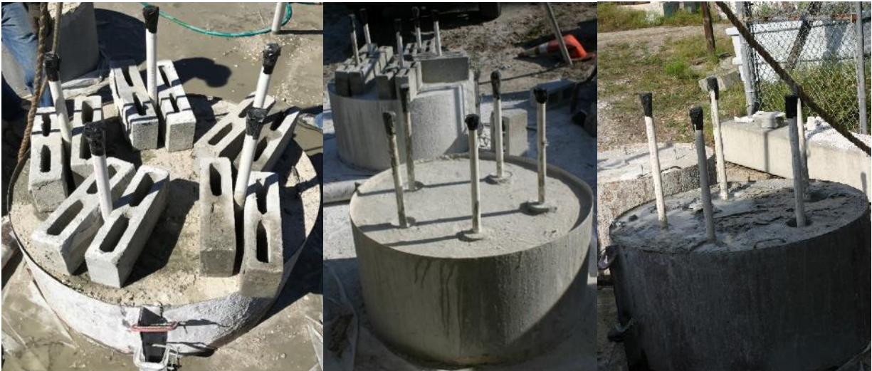
Figure 4.17. Sockets immediately after concreting (left), ready for load testing (center and right).
