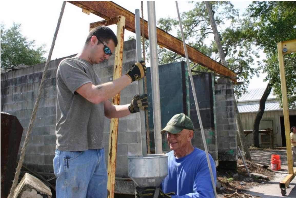
Figure 4.15. PVC tube containing the all-thread rod being pushed into the fresh concrete.
