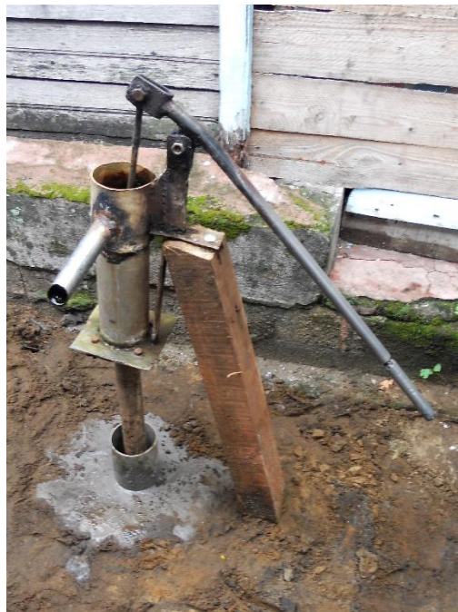
Figure 3.4 Concrete well apron constructed in this study. (Photo taken by the author.)
