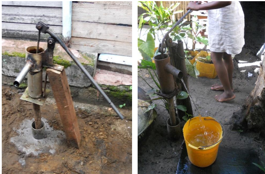
Figure 4.14 Left: The 50-cm diameter concrete apron is at the base of the pump. The wider diameter, shorter pipe coming out of the concrete is the pipe collar. Right: The pipe collar is the grey PVC pipe at the base of the pump. This is installed directly into the soil.
