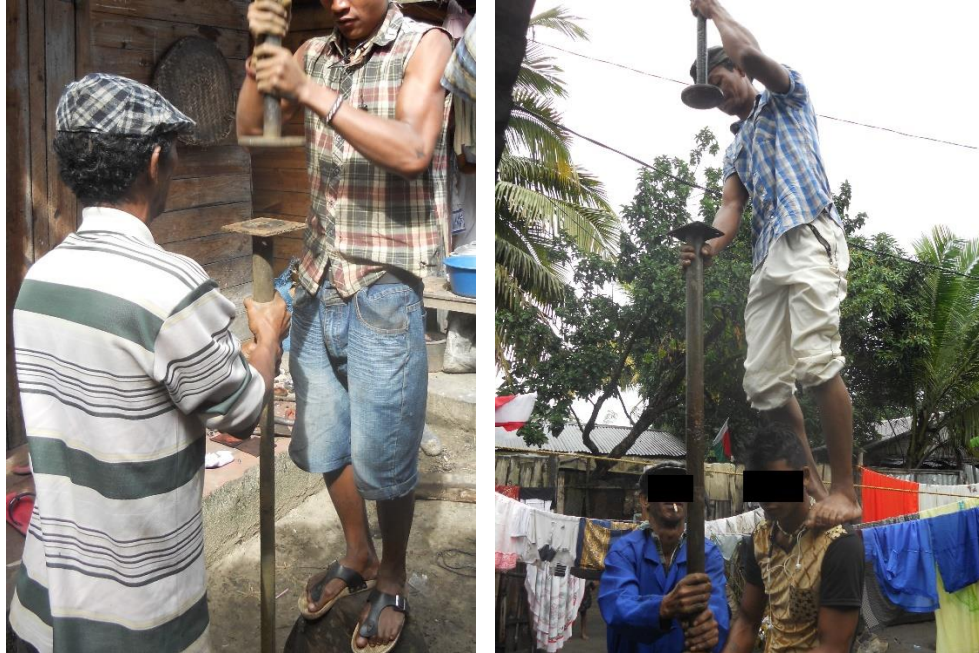
Figure 1.5 Malagasy Pitcher Pump technicians hammering a rising main into the aquifer. Right: Example of a case where the pilot hole collapsed before installation and the top flange was too high to be easily hammered in without standing on another technician's shoulders. This also shows the construction challenge when a well screen is being placed deeper than about 1.5 meters into the aquifer because any pilot hole dug below the water table will collapse in the same fashion. Left: Example of the normal case where a rising main is not being placed very deeply into an aquifer and is also being placed into a pilot hole that has not collapsed. (Photographs by the author.)
