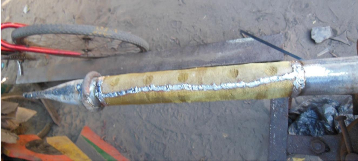
Figure 1.4 Well point and well screen made from a brass mesh soldered on with a leaded solder. (Photo by the author.)
