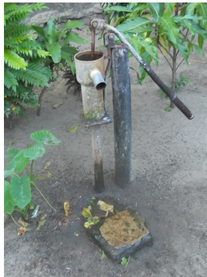
Figure 3.2 Example of Pitcher Pump in Tamatave without well head protection. (Photo taken by the author.)
