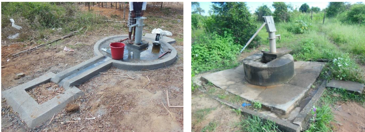
Figure 2.2 Left: A newly completed well apron for a community water supply with a hand pump being installed on a borehole in rural Madagascar. The apron is designed to drain spilled water away from the well pump and to a soak pit in the lower left of the image. Right: Damaged and cracked well apron on a hand-dug well. The well has been opened because the pump is not operating. (Pictures taken by the author.)
