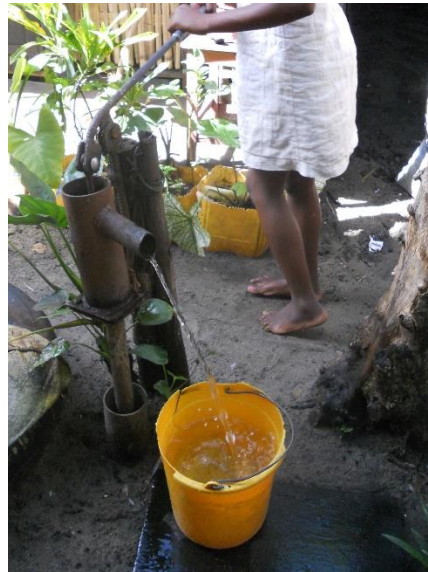
Figure 3.3 Example of a Pitcher Pump with pipe collar installed. (Photo taken by the author.)
