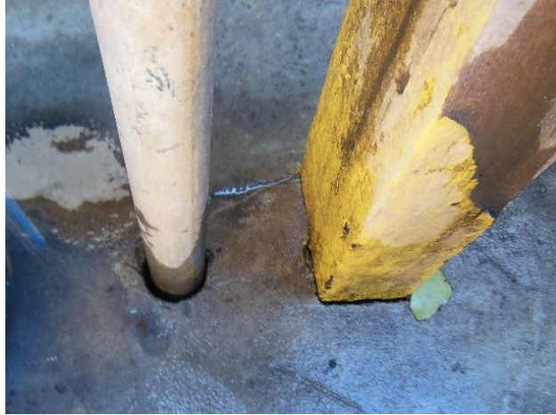
Figure 2.7 Example of the gap formed on a concrete well apron from deflection of the rising main during pumping. The rising main is the pipe on the left of the photograph. (Picture taken by the author.)
