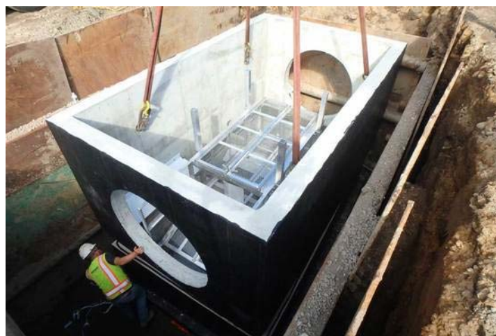
Figure 2-2: Baffle box retrofitted with screens (From www.suntree.com )
