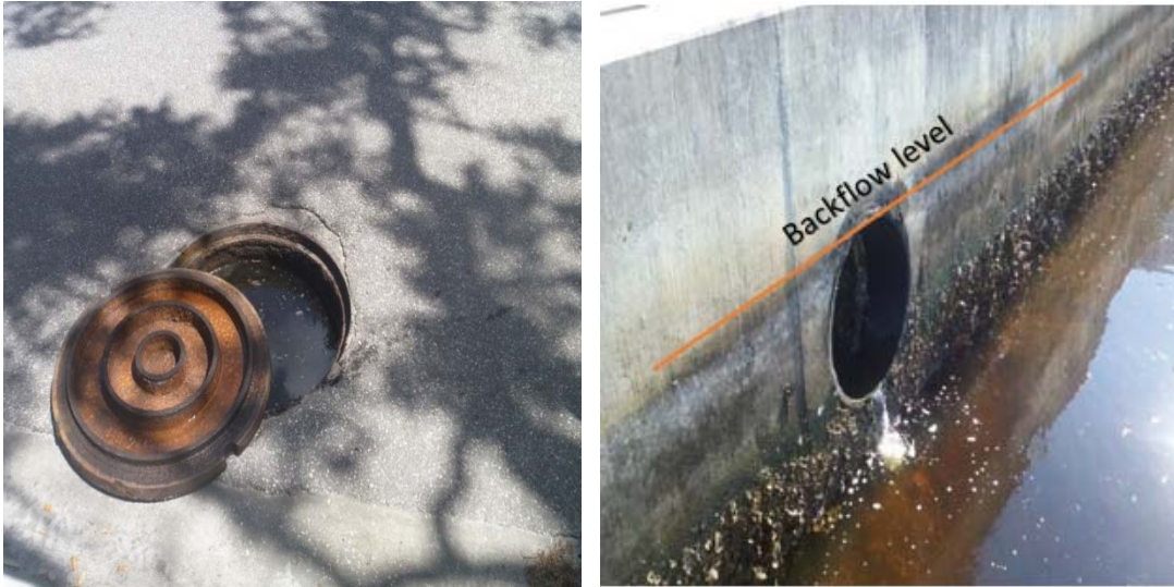
Figure 4-4: Stormwater units experiencing inundation (left) and tidal backflow (right)
