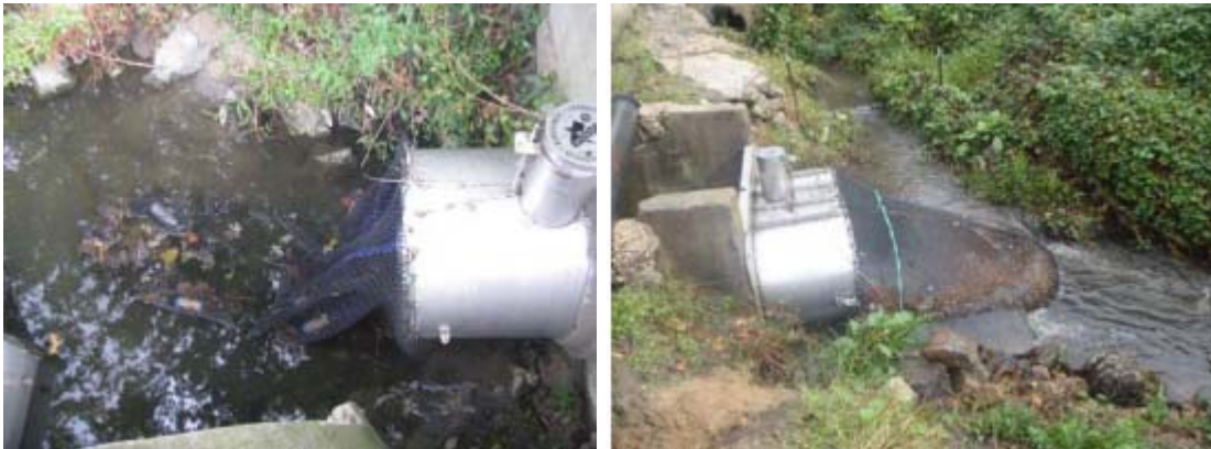
Figure 2-4: Bag filters installed in the Tred Avon Watershed Talbot County, MD (from Stack et al. (2013))
