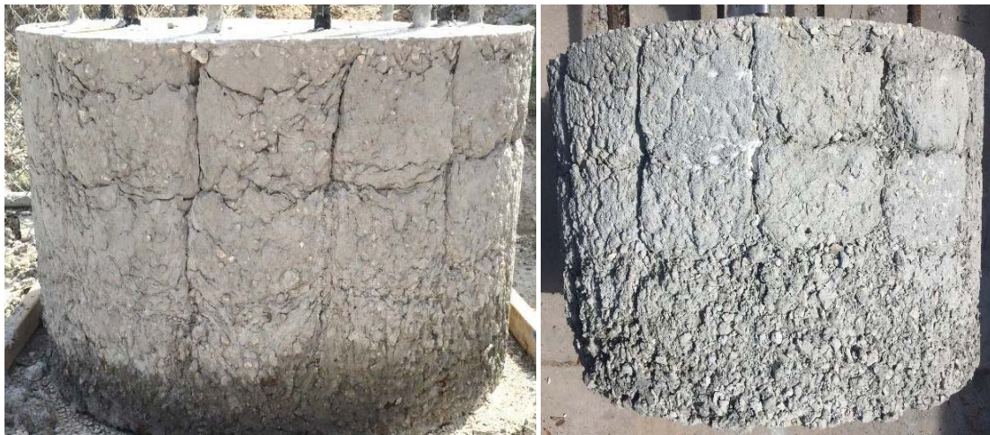
Figure 2.27 Shaft 21: f'c 4100 psi; drilled shaft mix, 42 sec/qt bentonite, coarse with well-defined creases
