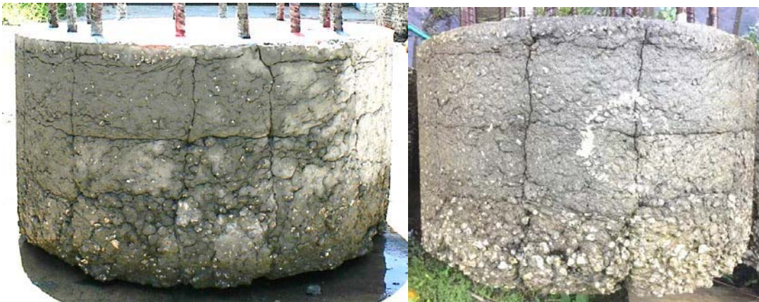
Figure 2.11 Shaft 5: f'c 4358 psi; drilled shaft mix; 90 sec/qt bentonite; coarse with well-defined creases.
