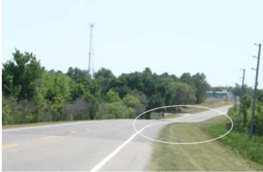
Figure 4.3. Visible subsidence along SR 33 approaching from the north.
