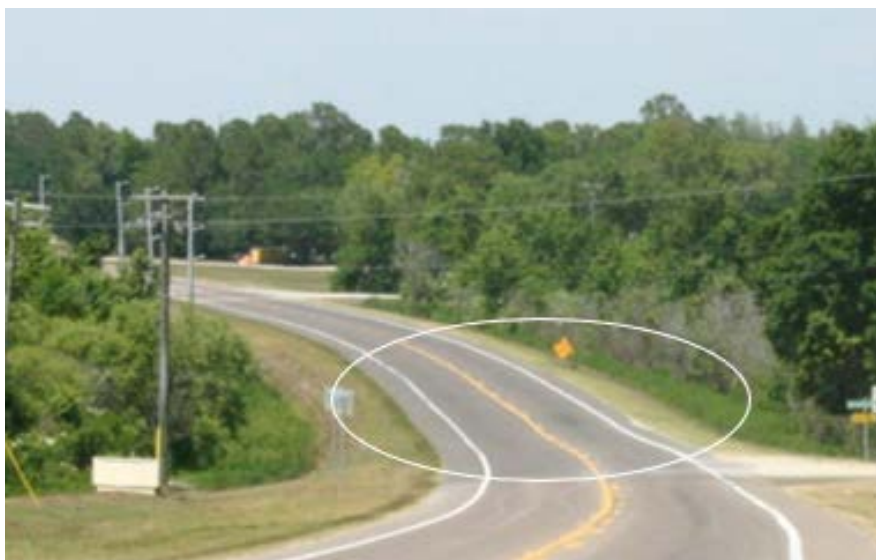
Figure 4.2. Visible distress along SR 33 approaching subsidence zone from the south.
