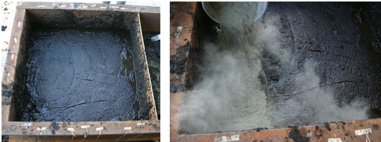
Figure 3.17. Right before cement was added (left), the initial addition of cement (right).
