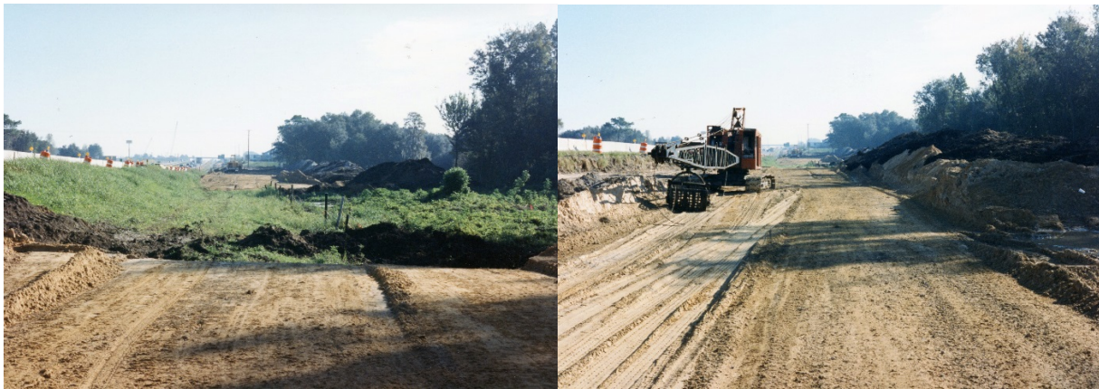
Figure 1.1. Organic soil replacement along Interstate I-4 between Tampa and Plant City, FL.
