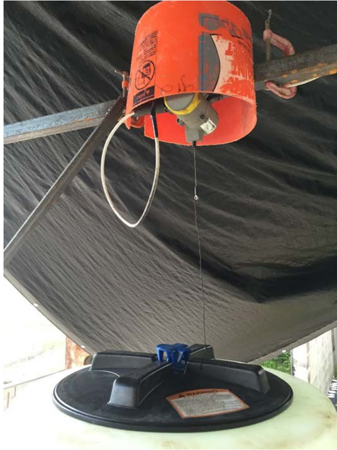
Figure 3.25. String line transducer above water tank (Baker, 2015).
