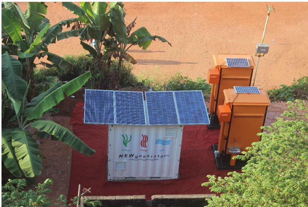
Figure C4: Overhead view of the site as installed during the initial month of testing for Chapter 6.
