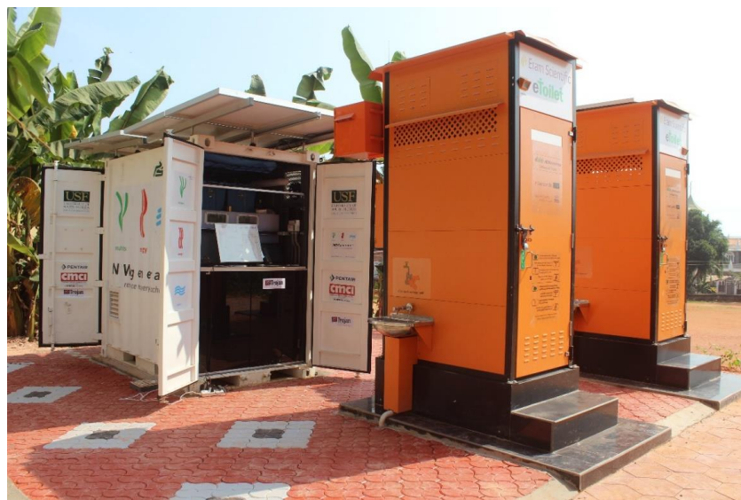
Figure 6.2: Site picture showing final system as installed at the site. The two orange eToilets can be seen with their associated sinks. The AnMBR housed in a shipping container and PV system can also be seen. In the background the playing field can also be seen.
