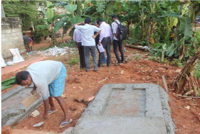
Figure C3: Site preparation and civil work prior to TRL 7 installation. The foundations for the eToilets as they were installed.
