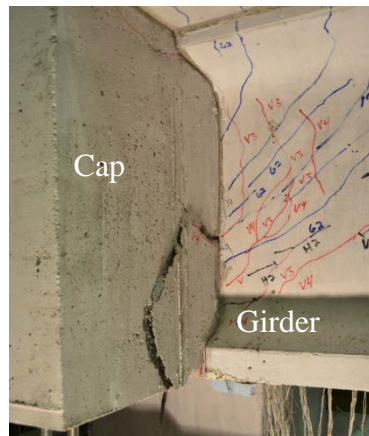
Figure 4.16: Spalling of cap cover concrete
