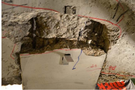
Figure 4.28: Spalling at bottom of girder to cap interface
