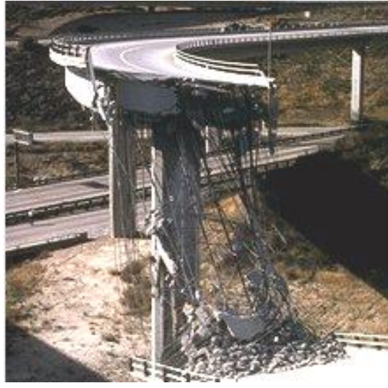
Figure 1.2: Bridge collapse during Northridge earthquake (USGS, 2010)
