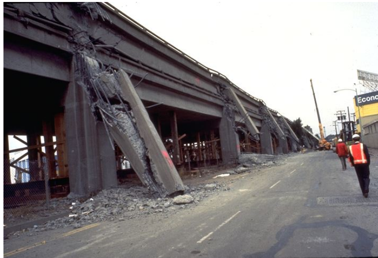
Figure 1.3: Damage to Cypress Street Viaduct in Oakland California (USGS, 1999)
