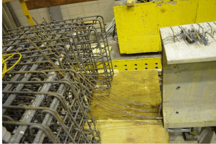
Figure 3.17: ESBF connection prior to cutting one strand and inserting strands into cap beam
