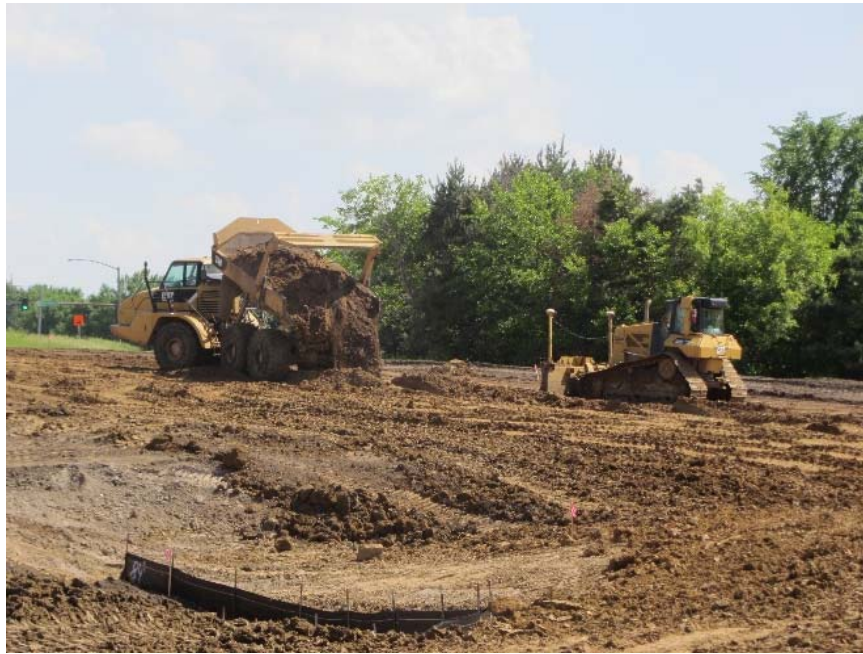
Figure 68. Caterpillar 740 dump truck used to place loose fill materials and Caterpillar dozer was used to spread loose lift material
