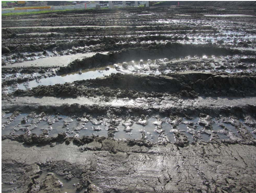
Figure 98. Seepage occurred in the construction site
