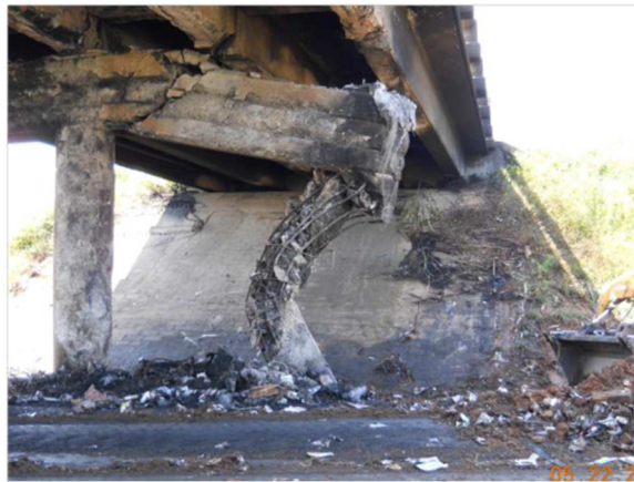
Figure 2. Resulting damage caused by the tractor-trailer collision with the SC Highway 150 bridge over I-85 (Kudelka 2011)
