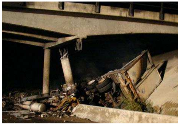
Figure 1. Pier support failure caused by tractor-trailer impact in Grand Junction, CO (Gallegos and McPhee 2007)
