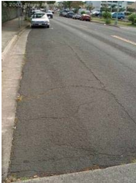
Figure 11: Block cracking, type of thermal cracking [21]
