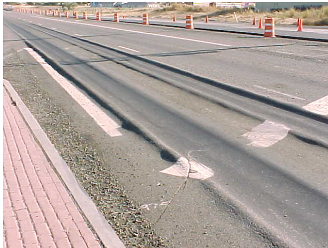
Figure 9: Severe rutting in flexible pavement [19]
