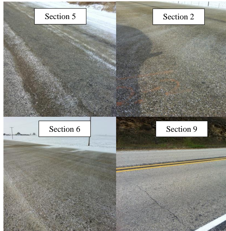
Figure 4.5. Surface Condition of Chip Seals
