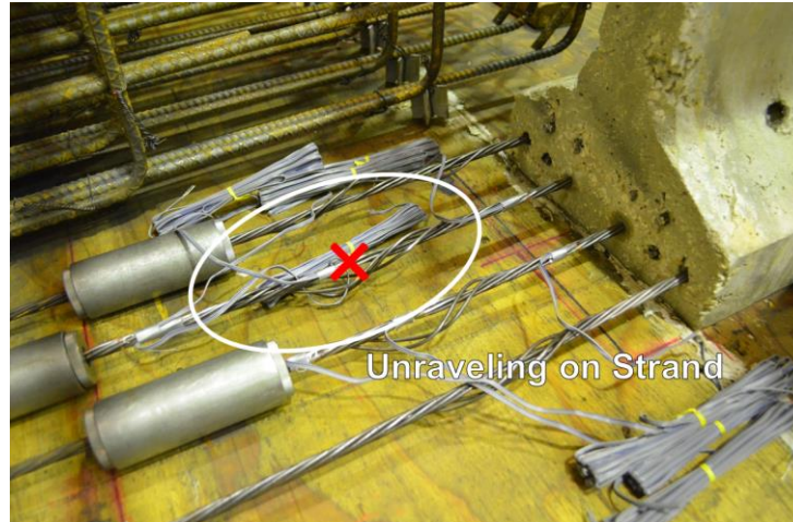
Figure 4-14 Placement of Strain Gauge on Unraveled Portion of a Strand in the ESMS Connection
