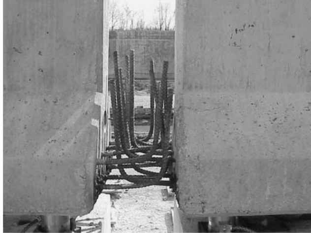
Figure 2-15 Congestion within Connection Region due to the Use of Bent Bars (Miller et al., 2004)
