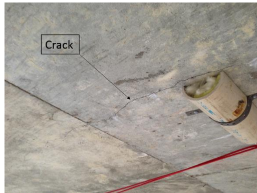
Figure 45. Relative position between crack and strain gauge in the fifth bay
