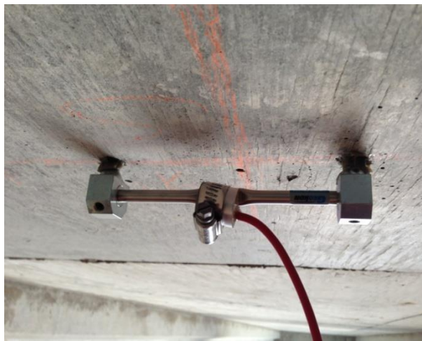
Figure 16. Vibrating wire strain gauge at the bottom of deck
