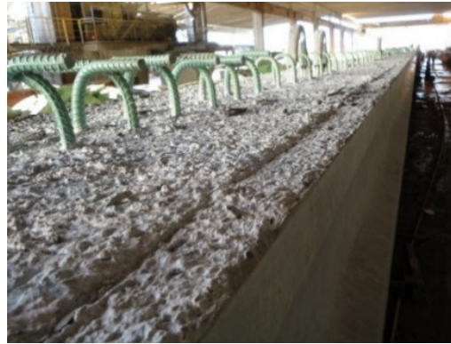
Inconsistent troweled surface along the length of a PPCB
