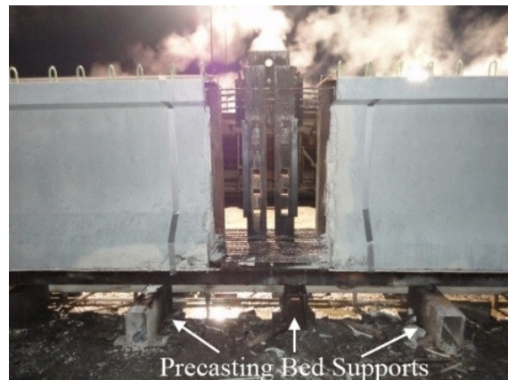
PPCB ends between the bed supports
