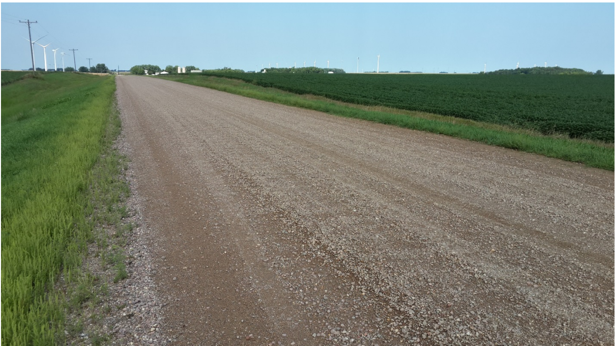
Figure 22 Jackson County Road 76 Surface Conditions in August, 2013 (Photo by the Author)
