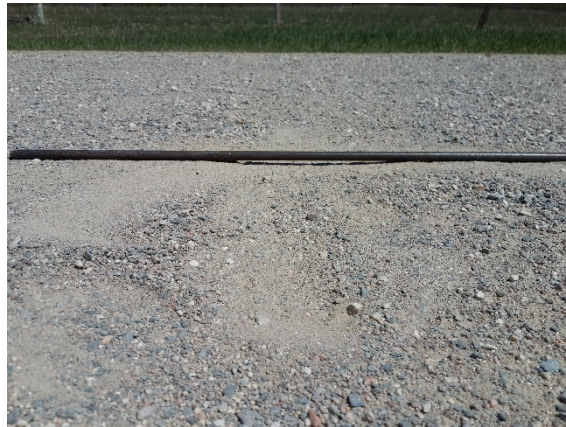
Figure 61 Typical Corrugation in the South Section/3rd Section (Photo by the Author)
