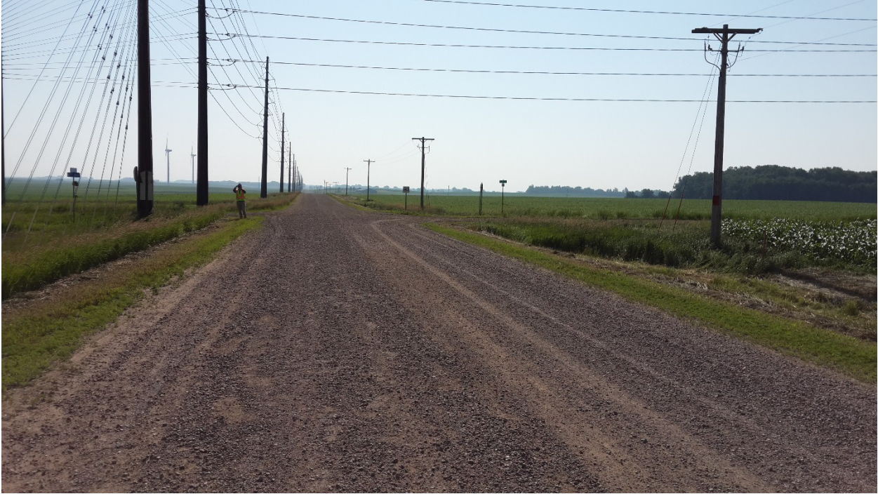
Figure 21 Jackson County Road 76 Surface Conditions in July, 2013 (Photo by the Author)
