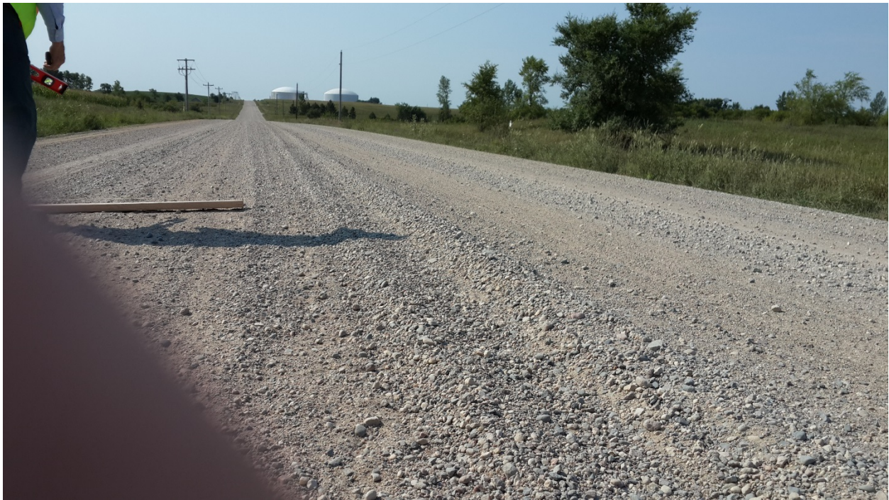
Figure 20 Loose Aggregate on CR 35, Pope County (Photo by the Author)
