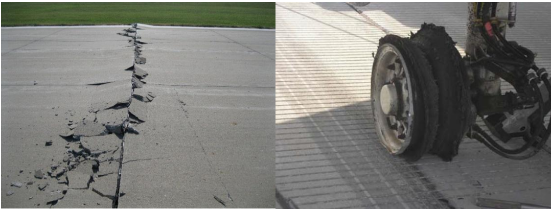
Figure 2-5. Pavement blowup and damaged aircraft in Ankeny Regional Airport runway (photo courtesy of Snyder & Associates, Inc./Polk County Aviation Authority).
