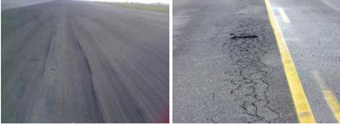
Figure 3. Airport Pavement Rutting (Left) and Potholes (Right) [8]
