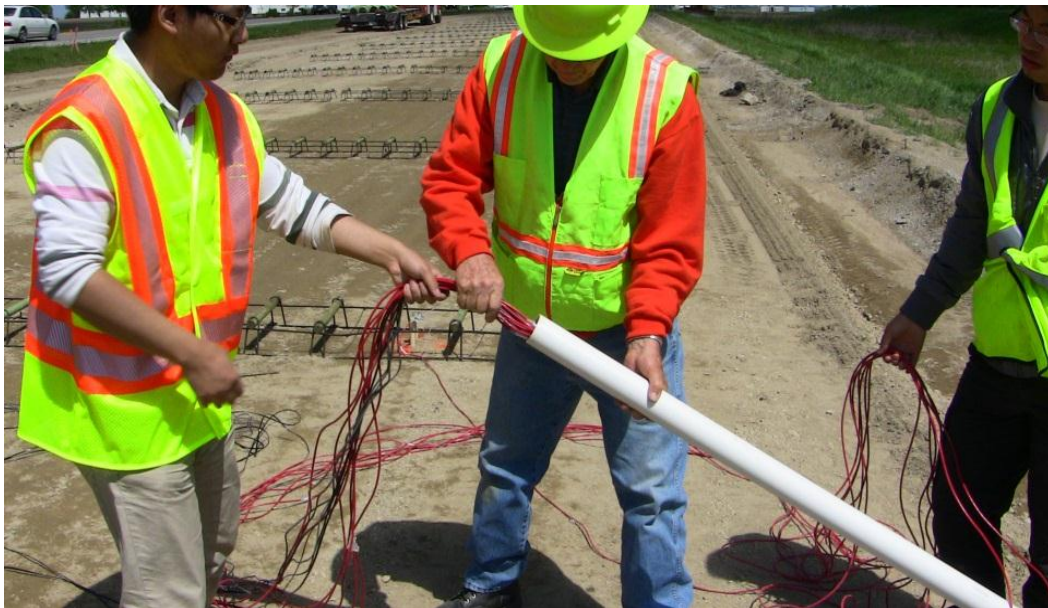
Figure 3-14. Wires in PVC pipe.
