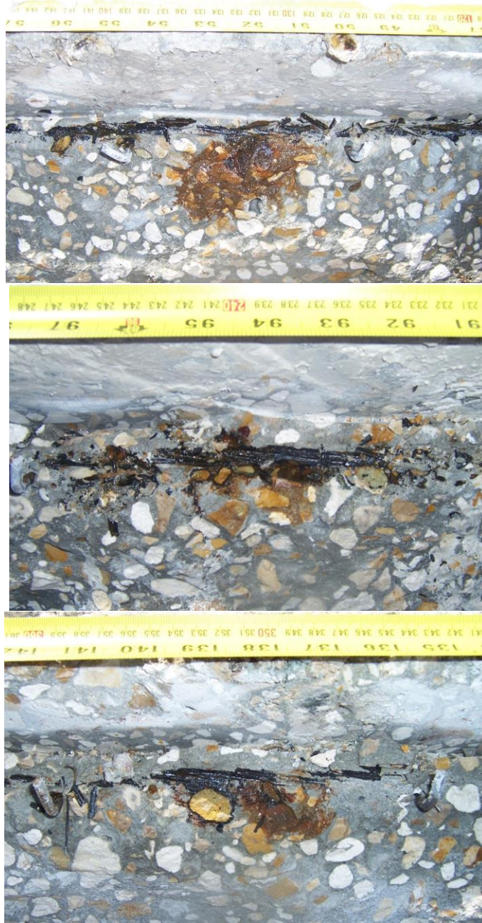
Figure 21. Three different instances of localized corrosion. (Bridge B) Note that the measurement datum for the indicated distances was the waterline.
