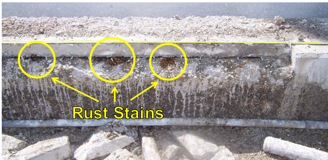
Figure 20. Exposed strand in region nearest waterline of autopsied pile. (Bridge B) Note rust-colored regions. (Photo taken immediately after strand was exposed.)
