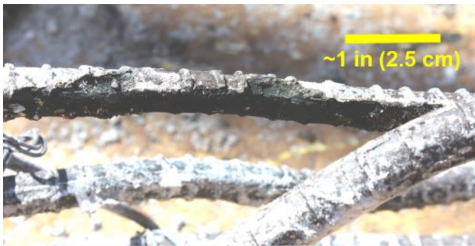
Figure 23. Locally corroded steel in region below mudline. (Bridge C) Note corrosion-related cross-sectional area decrease of bar near top of photo.
