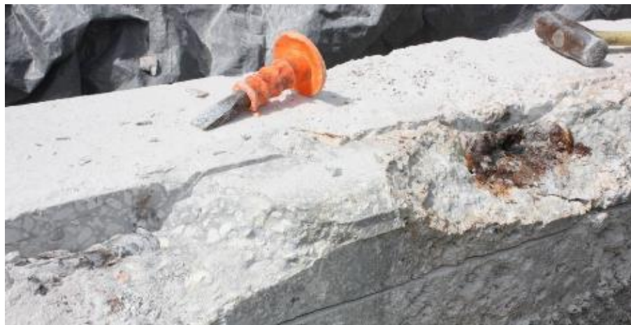
Figure 9. Rust stains in concrete cover observed during bar removal. (Bridge A Pile #2)
