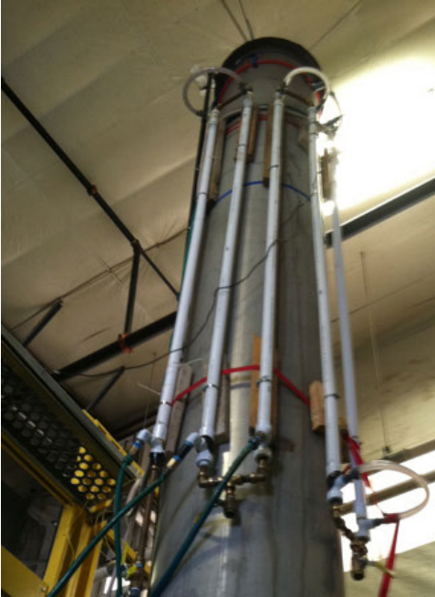
Heat exchanger attached to 1600L
