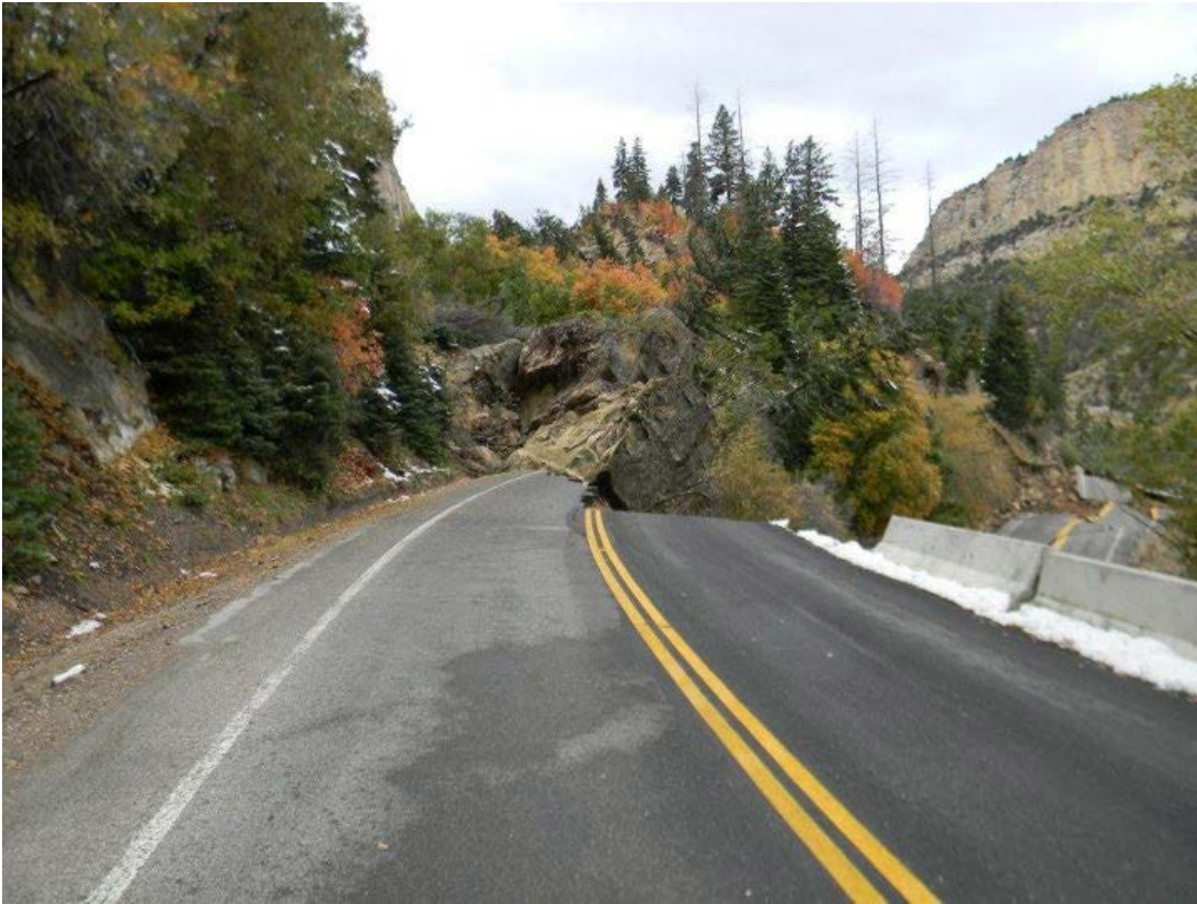
Figure C.20.1 Aftermath of Landslide on SR 14 (UDOT 2012)
