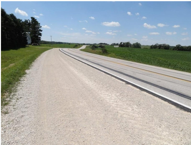
Figure 29. Shoulder of US 18 on eastbound near west of Clermont
