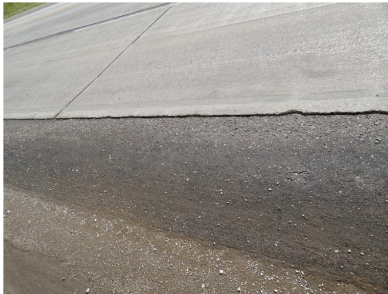
Figure 20. Southbound shoulder of US 169 south of Algona
