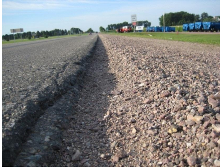
Figure 1. Edge rutting on granular shoulders (by Thang Phan)
