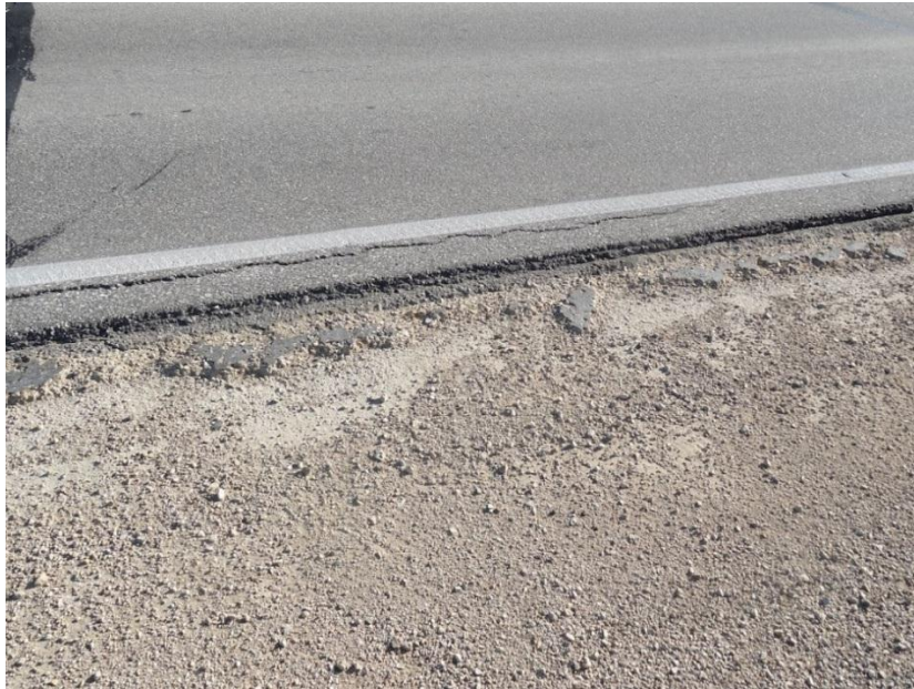
Figure 26. Soapstock missing near east of Allison
