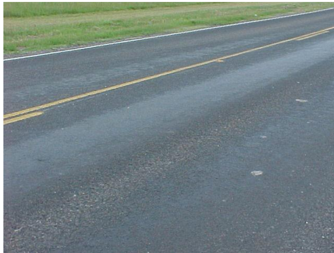
Figure 31: Bleeding Chip Seal (Webb 2010)
