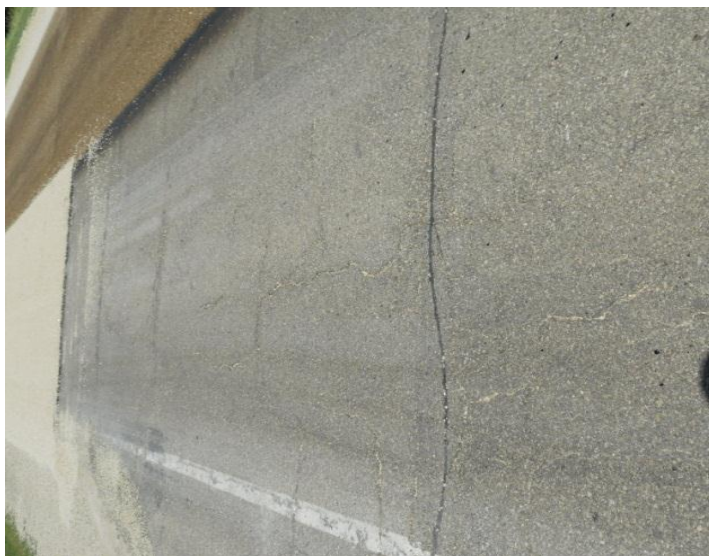
Figure 6: Road With Minor Cracks (photo taken by author)
