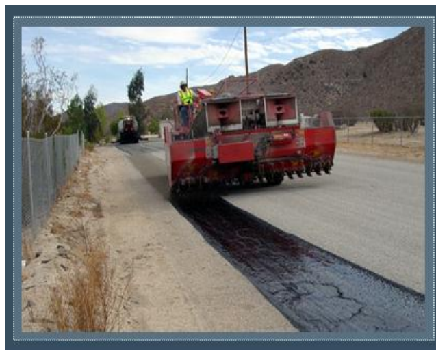
Figure 41: Fog Seal Poor Practice (NHI PPTCG 2007)
