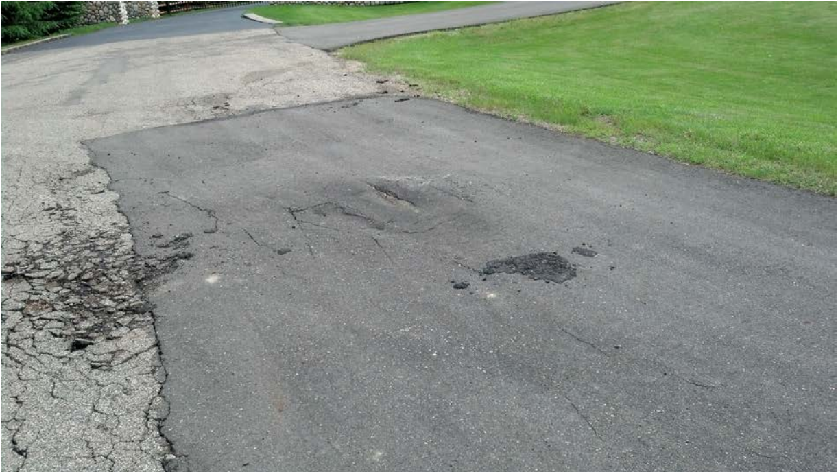
Figure 13: Picture to show failure modes of Schurman Drive-Picture by Francis O. Dayamba
