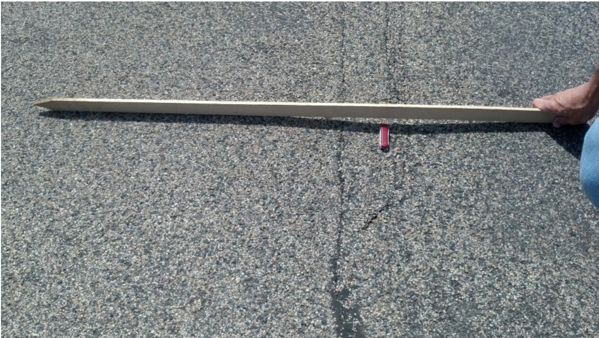
Figure 28: Example of transverse cracking on CSAH 14-Picture taken on 8/14/13 by Francis Dayamba
