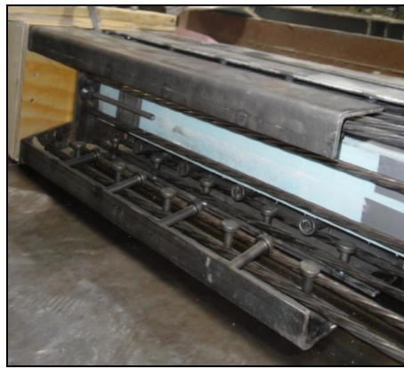
Figure 5-11: A UHPC Pile Splice Installed at One of a the UHPC Pile Formwork
