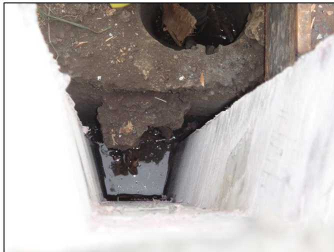
Figure 5-40: Void that Formed from Installation of P3
