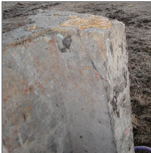
Figure 5-26: Slight Damage observed to P3 Pile Head after Driving the Pile in Place
