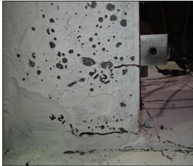
Figure 4-22: Hairline Tensile Cracks that Developed on the UHPC Pile in UPAC-2 at the 12 kip Lateral Load Step with a 100 kip Axial Load
