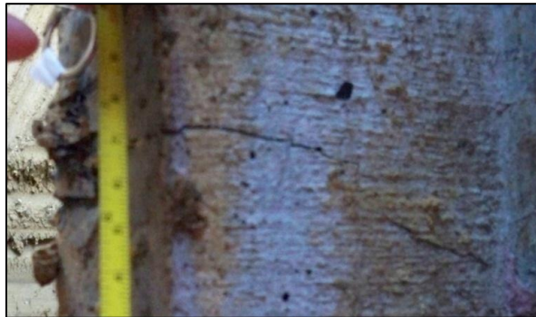
Figure 5-54: A Flexural Crack Found at a distance of 9 ft. from the Ground Surface on P4 due to the Lateral Load Test
