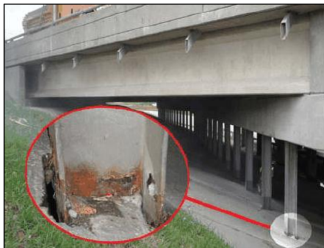
Figure 1-6: Corroded Steel H-Pile (Ehsani et al. 2012)
