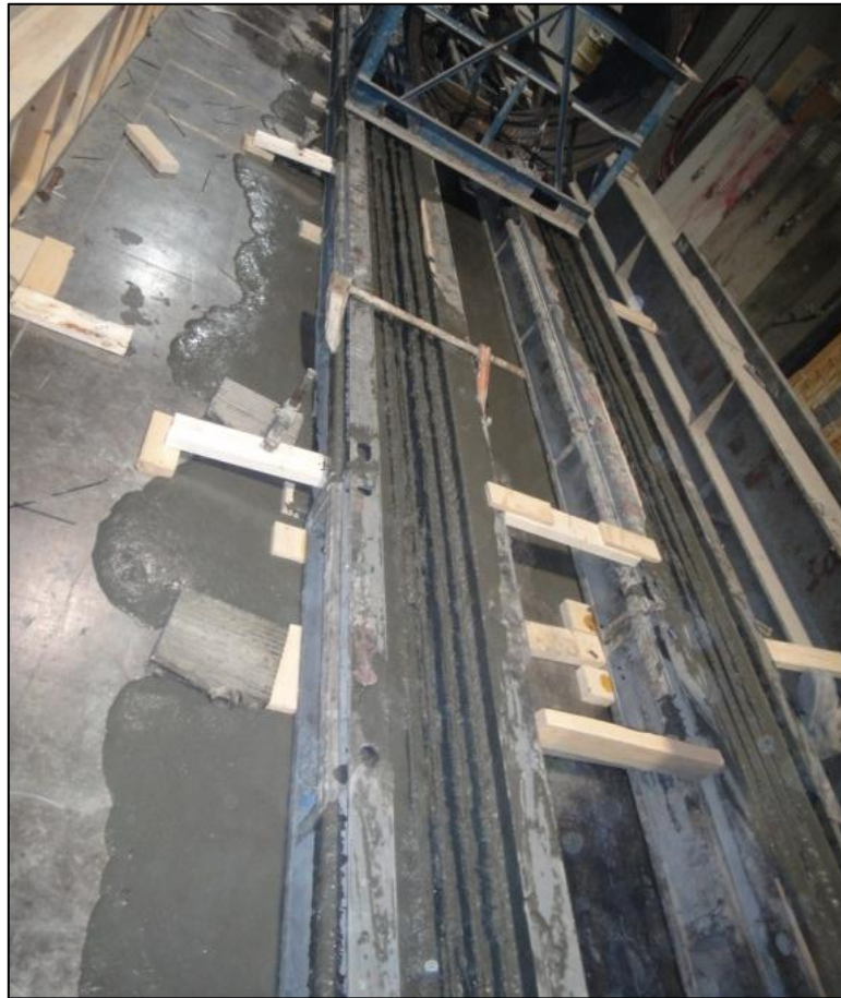
Figure 5-16: Steel Forms Beginning to Tilt Causing UHPC to Leak
