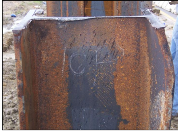
Figure 1-5 Damage to Pile Head at End of Driving (Ng et al. 2011)
