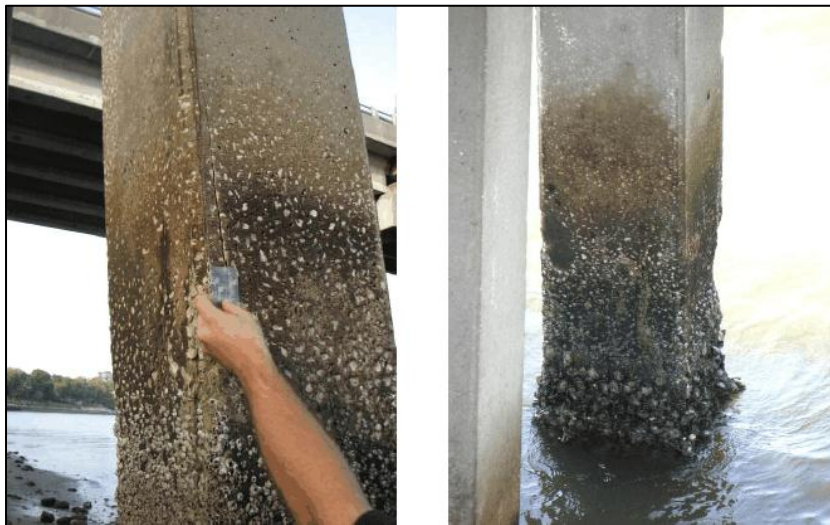
Figure 1-3: Damage to Prestressed Concrete Pile Due to Corrosion (Moser et al. 2011)
