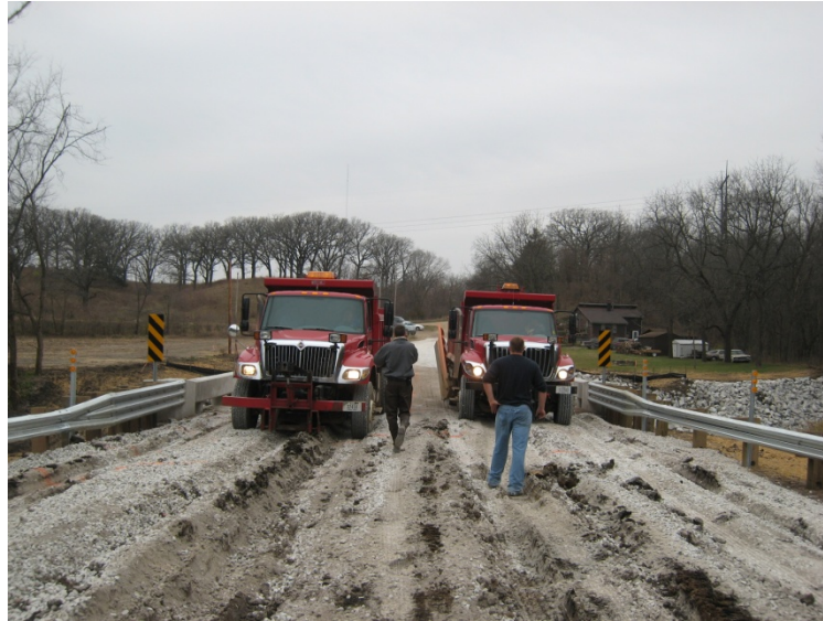
Figure 5-106. Rutting of bridge approaches due to live load testing.
