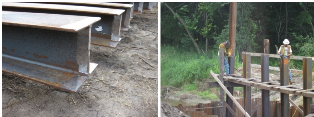
a.) Preparation of piles for welding b.) Welding two 40 ft sections together
