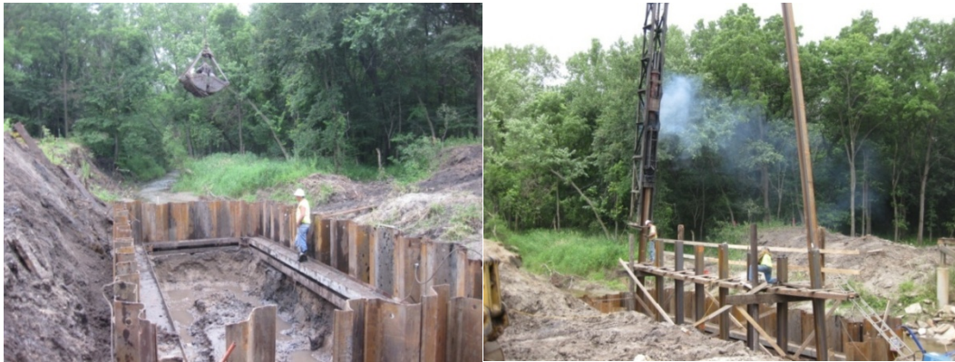
a.) Cofferdam placement and excavation b.) Placement and driving of battered piles
