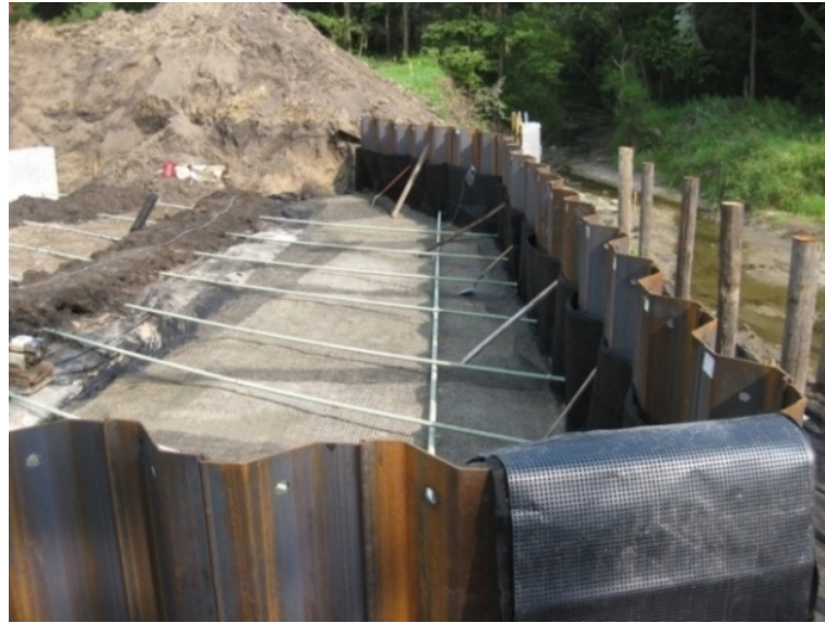
a.) Deadman and tie rods anchoring the west abutment sheet pile wall
