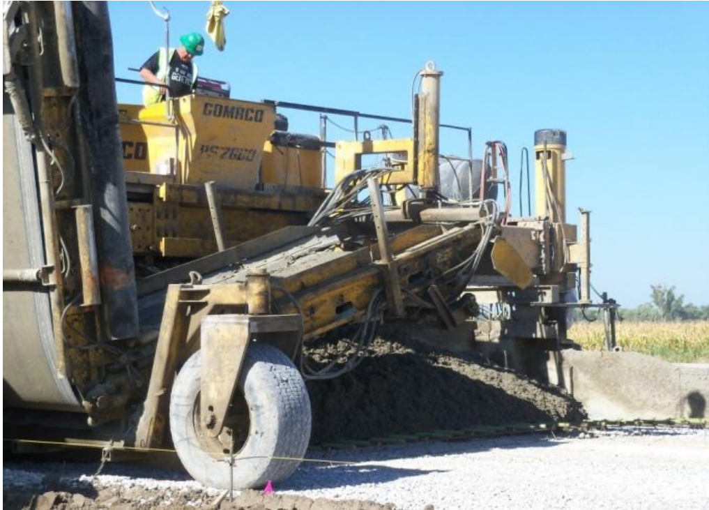
Figure 7 Concrete being dumped into a belt placer and spread by the placer.
