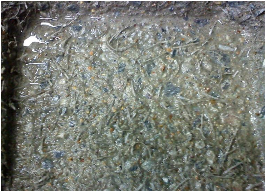
Figure 21 NH salt scaling sample after 50 th freeze-thaw cycle.
