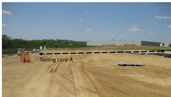
Figure 53. DCP-CBR profiles on testing lane A – unpaved area granular subbase (from White et al. 2009)
