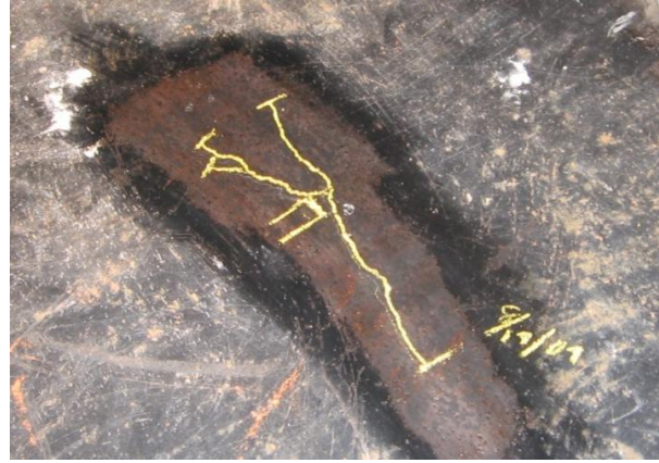
b. Close-up of top web plate cracking
