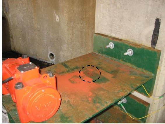
a. Overview of Top Web-Plate Cracking
