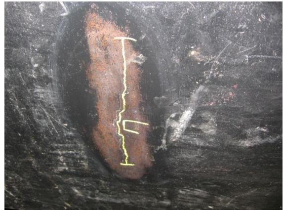
d. Underside of bottom web plate cracking
