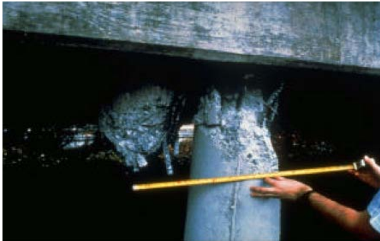
(b) Flexural shear failure of pile to bent connection
