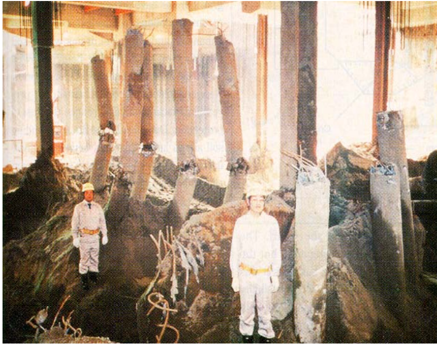
Figure 1.5. Piles supporting the NHK building sheared by lateral spreading during the 1964 Niigata earthquake (Hamada, 1991)
