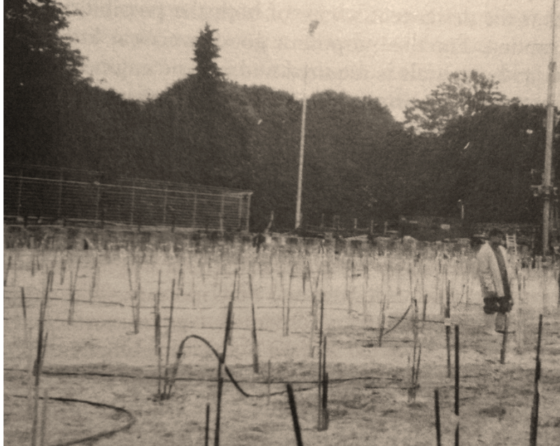
Figure 2.2 Single port grout pipes used in the foundation work for the new Offices of the German President of State (Semprich and Stadler, 2002)
