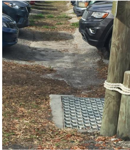
Figure 2.1 Asphalt parking swale demonstrating the typical construction configuration for commercial parking lots (Rushton & Hastings, 2001)
