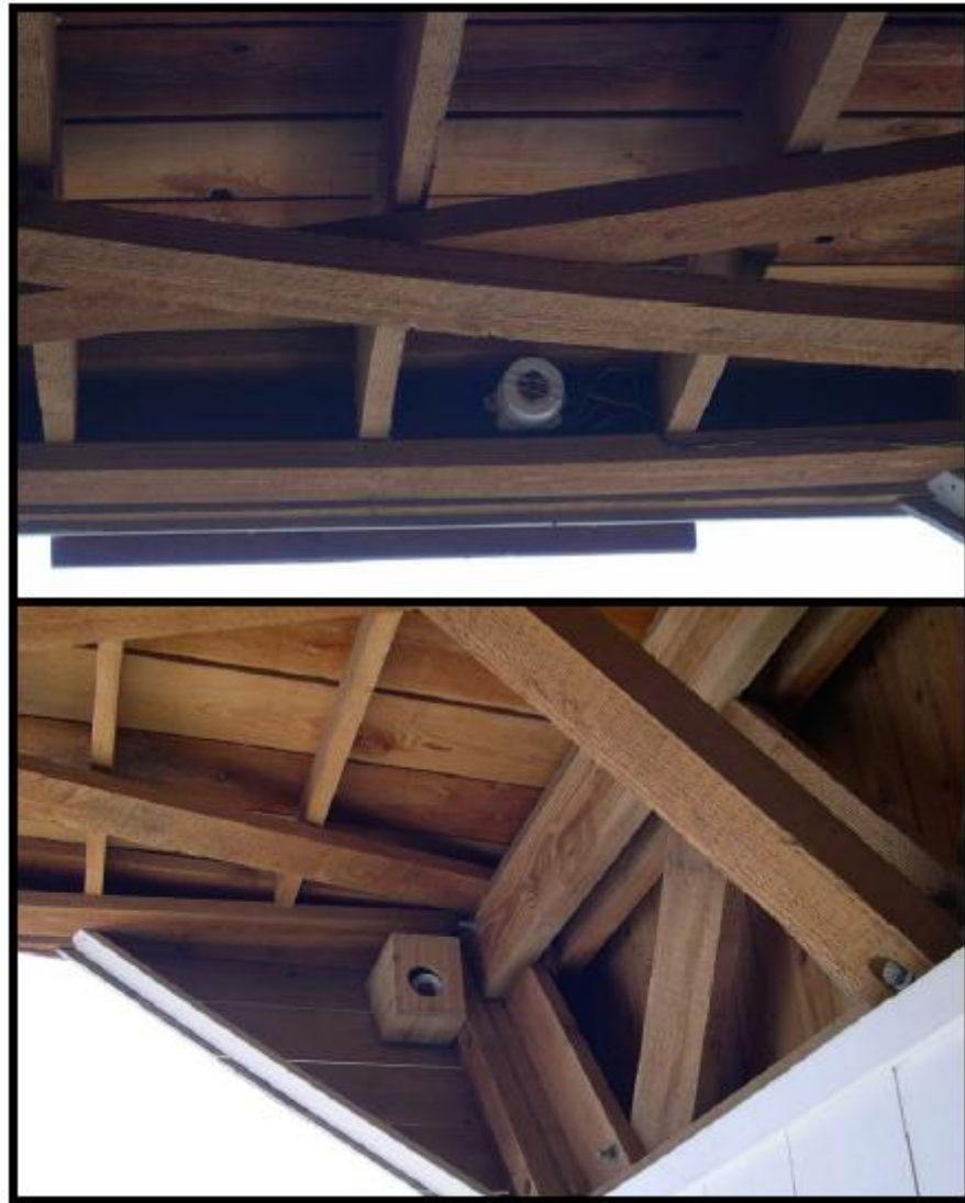
Figure 9: Flame Detector in Covered Bridge without Encasement (top) and With Encasement (Bottom)
