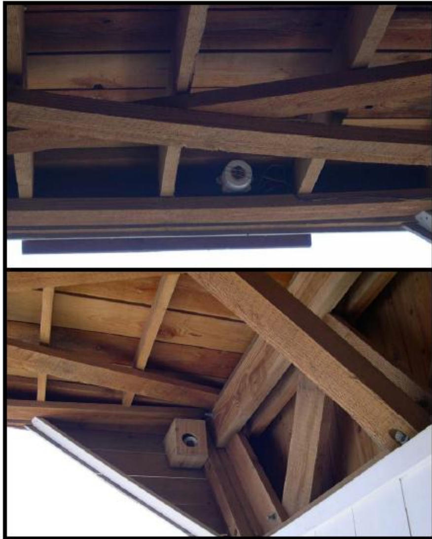
Figure 64: Flame Detectors with and without Wood Coverings
