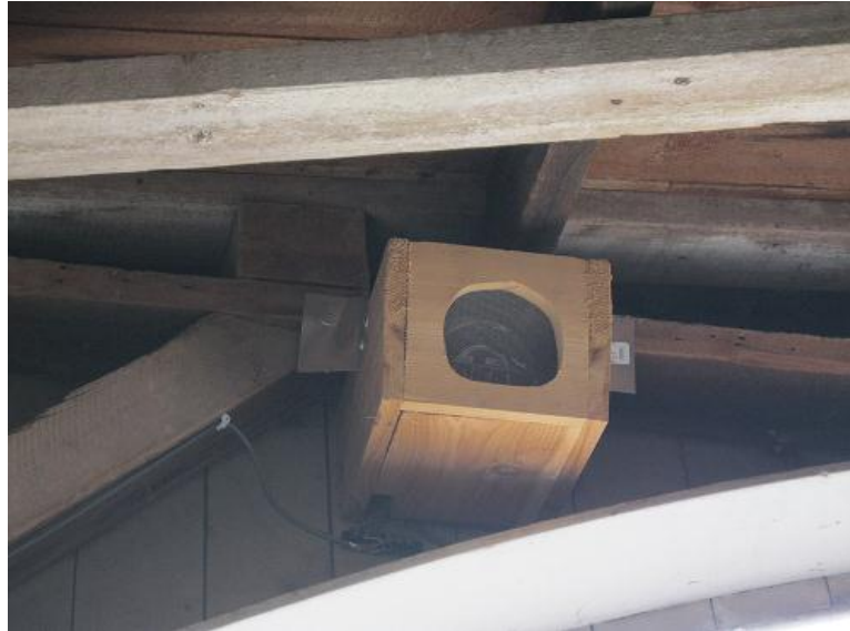
Figure 54: Flame Detector Prior to Alarm
