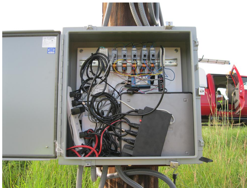
Figure 62: Inside of Typical NEMA Enclosure
