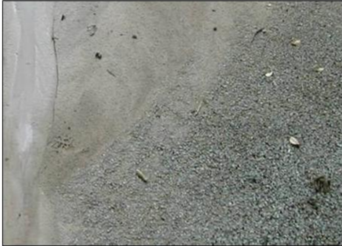
Figure 2-22. Clogging Failure Caused by Construction Runoff
