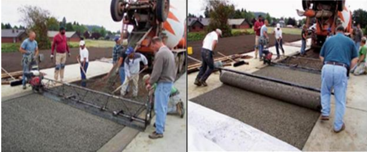
Figure 2-16. Compacting Pervious Concrete Using Vibratory Screed (Left) and Weight Roller (Right) (Adopted from [54])
