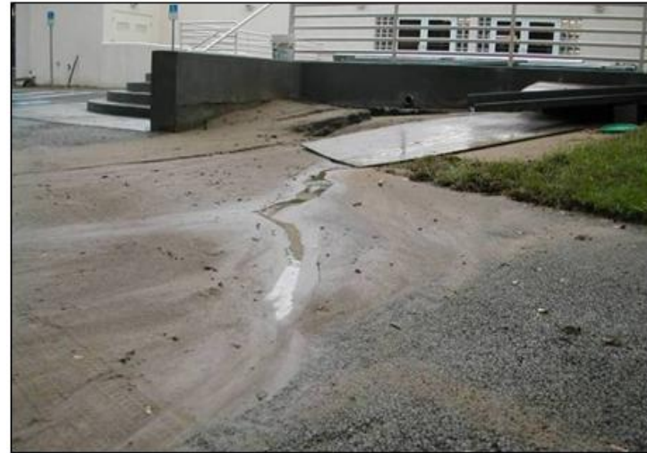
Figure 2-21. Clogging Caused by Surrounding Unplanted Area
